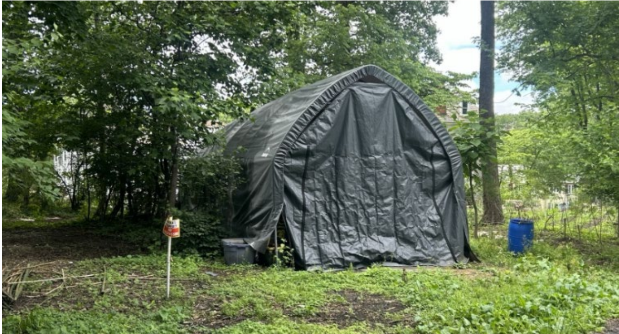
Figure 5: View of the accessory structure(s) from Hollow Glen Place (May 2026, Historic Preservation Division).
