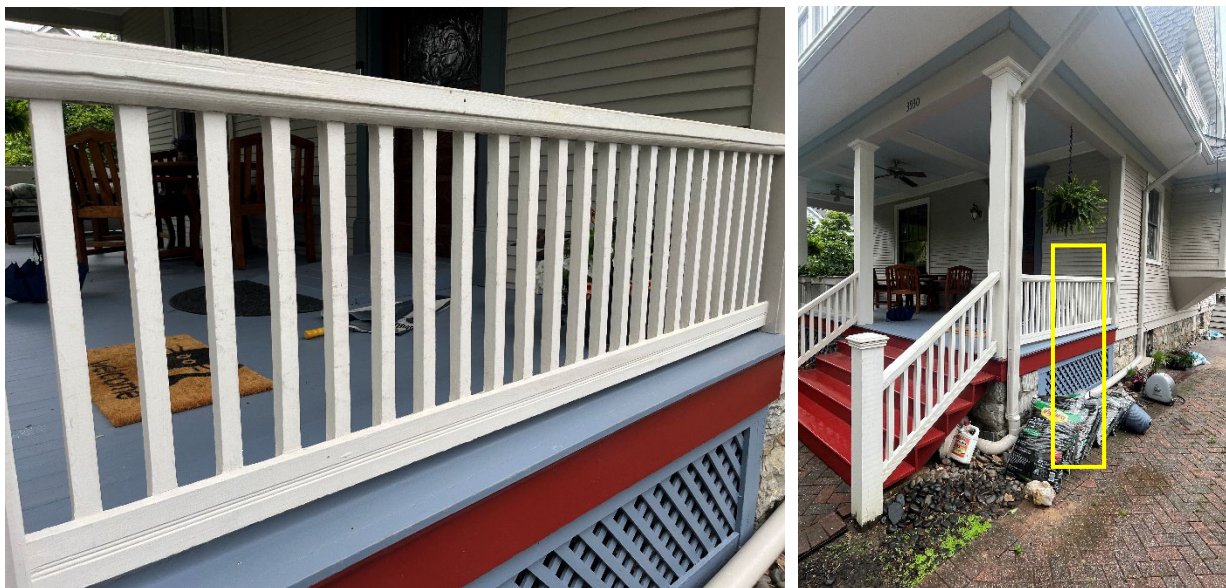
Figure 5: Detail of the existing railing (left) and view of the porch with approximate location of the proposed lift outlined in yellow (right).
