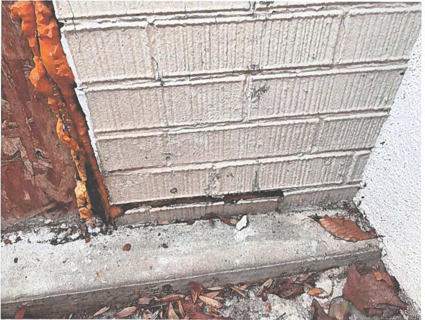
INSEL BACK CRACK
