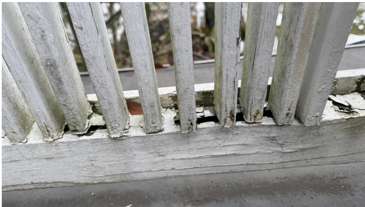
Figure 2: Detail of the existing second-floor railing condition.
