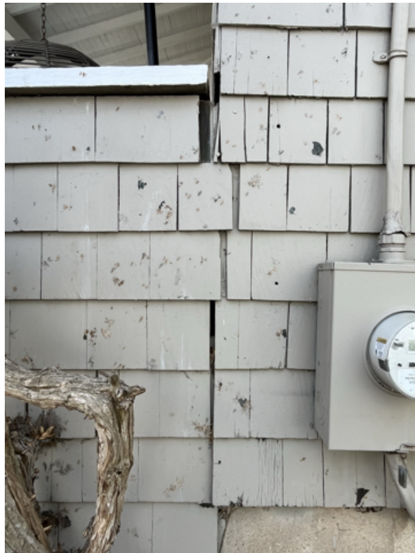
Detail: 6704 WESTMORELAND AVE. PORCH SEPARATION
