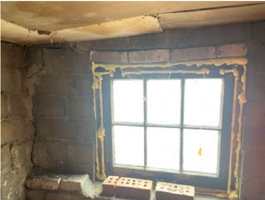
Detail: 6704 WESTMORELAND AVE. FAILING PORCH LINTEL
