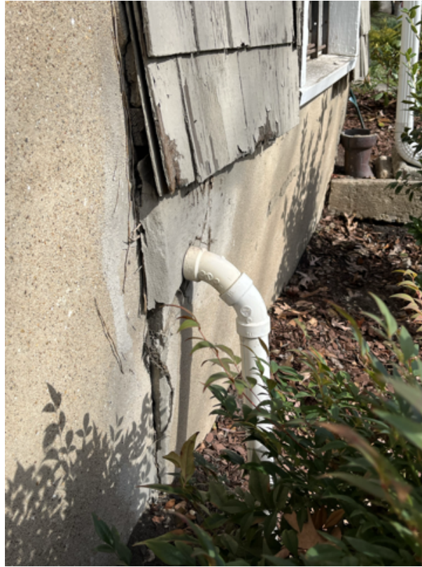
Detail: 6704 WESTMORELAND AVE. CRACKED PORCH FOUNDATION
