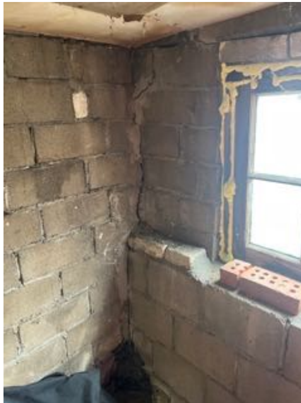
Detail: 6704 WESTMORELAND AVE. CRACKED PORCH FOUNDATION
