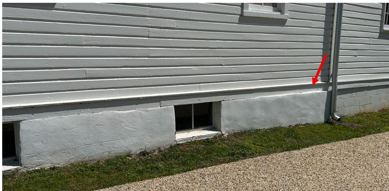
Figure 7: Location of the proposed louver on the west side elevation, shown with a red arrow. Evidence of previous patching of the bandboard is evident.
