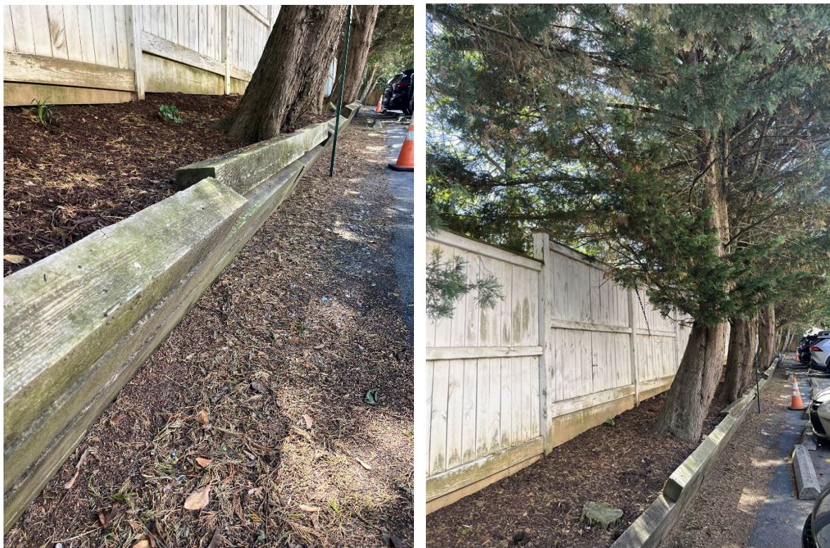
Figure 5: Retaining wall to be replaced (left) and fencing (right).
