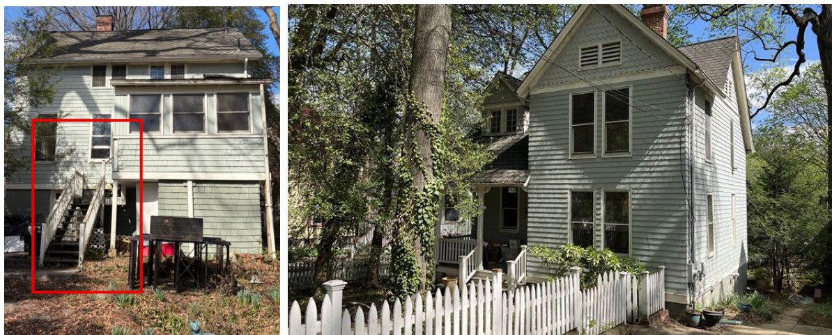
Figure 5: Rear view of the subject property with the existing stair indicated with a red box (left) and the subject property from the right-of-way, showing that the existing stair is not at all visible (right).
