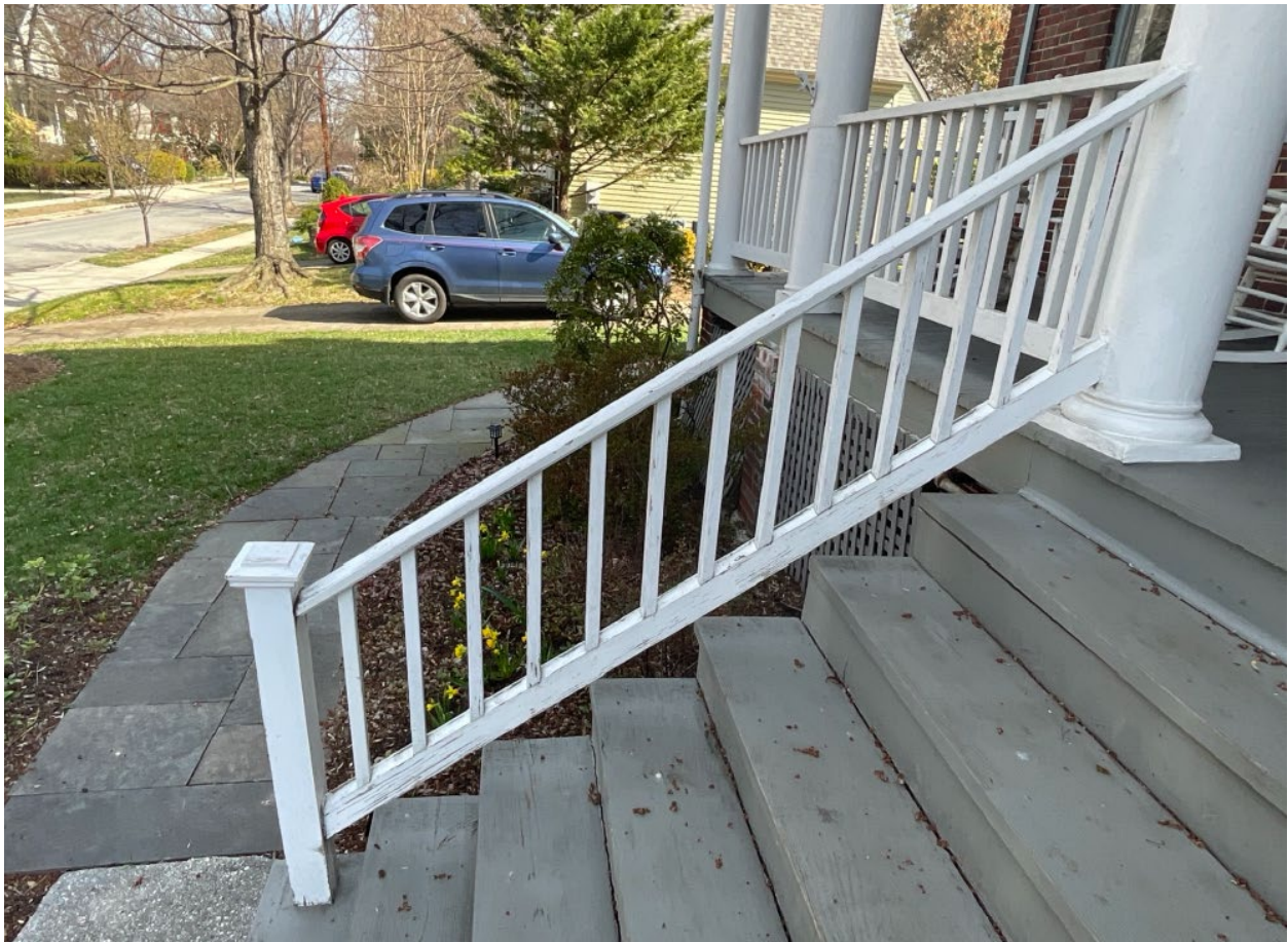
Figure 2: The existing railing is mounted on the bottom stair and abuts the existing wood column.
