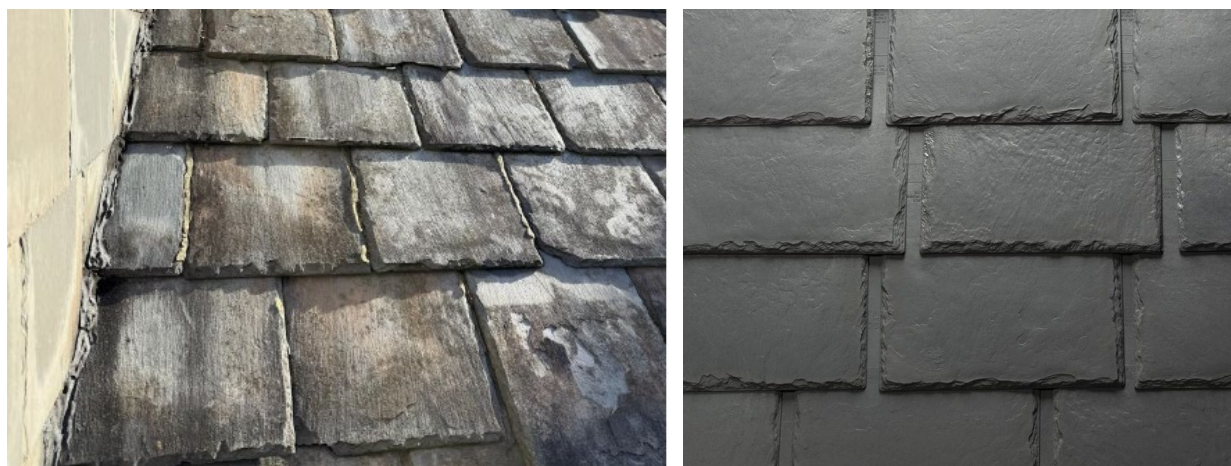
Figure 6: Detail of the existing slate roofing (left) and stock image of the EcoStar Majestic synthetic slate roofing (right).
