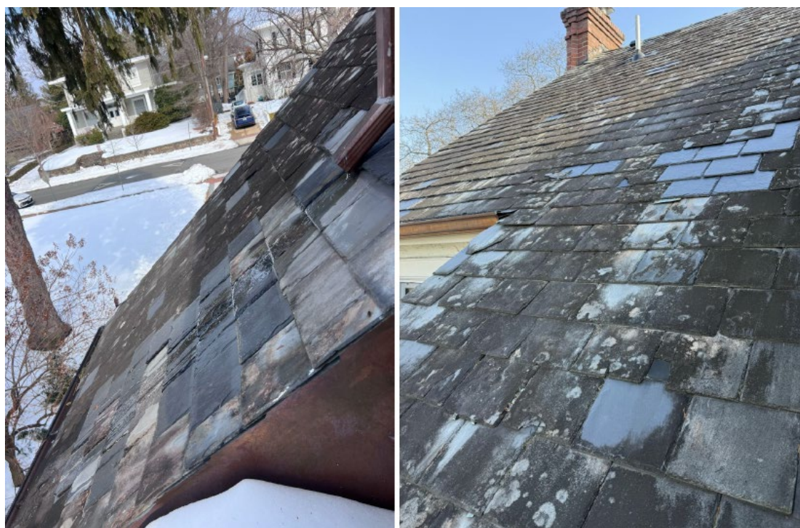
Figure 5: Detail of the existing slate roof showing the historic shape and color and areas of patching.
