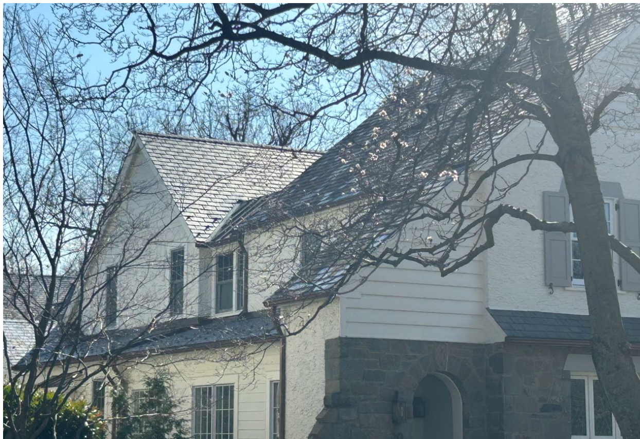
Figure 4: View of the juncture between the historic slate on the main block and the EcoStar Majestic synthetic slate on the non-historic rear addition (March 2026, Historic Preservation Division).
