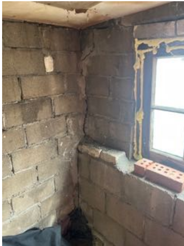
Detail: 6704 WESTMORELAND AVE. CRACKED PORCH FOUNDATION
