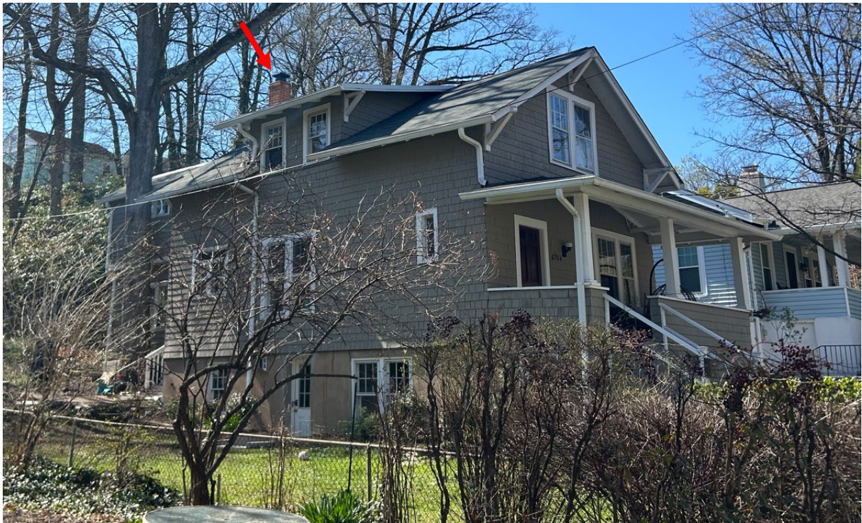
Figure 14: View of the front and southeast side elevations showing the chimney proposed for removal.
