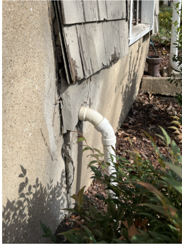
Detail: 6704 WESTMORELAND AVE. CRACKED PORCH FOUNDATION
