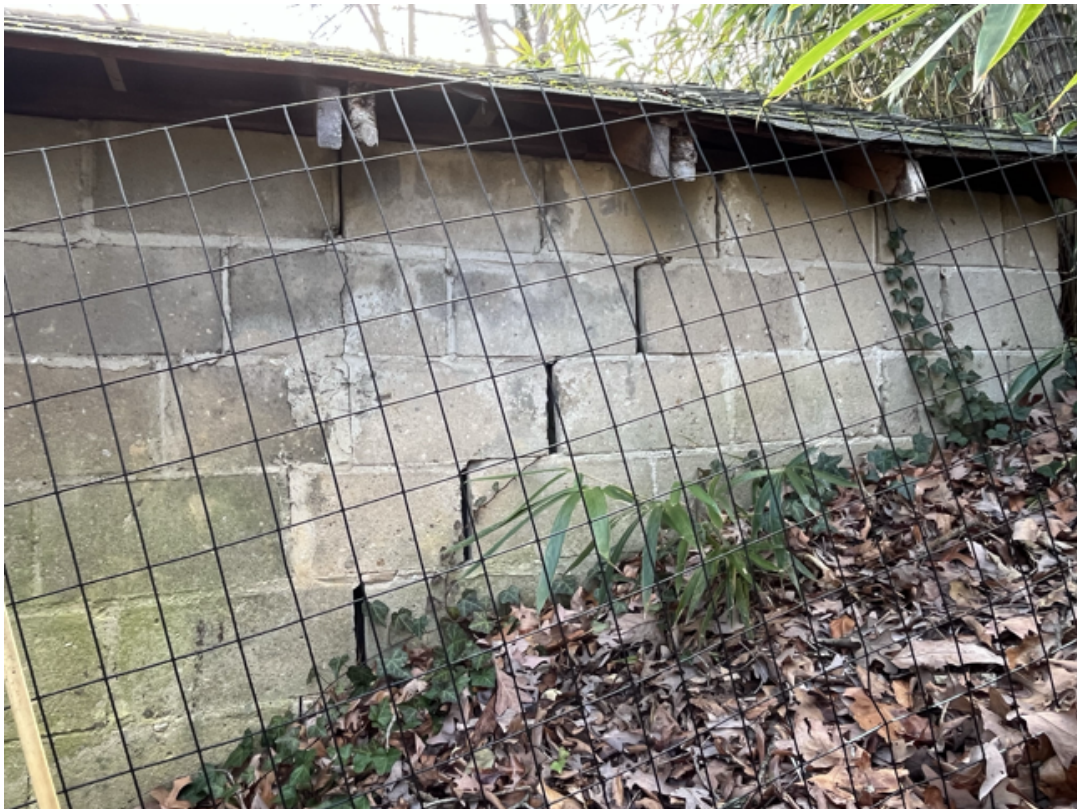
Detail: 6704 WESTMORELAND AVE. SHED CRACKED FOUNDATION
