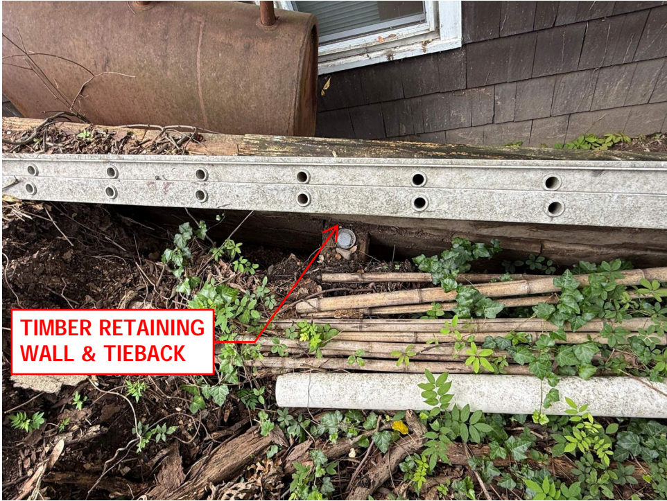
PHOTO 21: DISPLACED TIMBER RETAINING WALL
