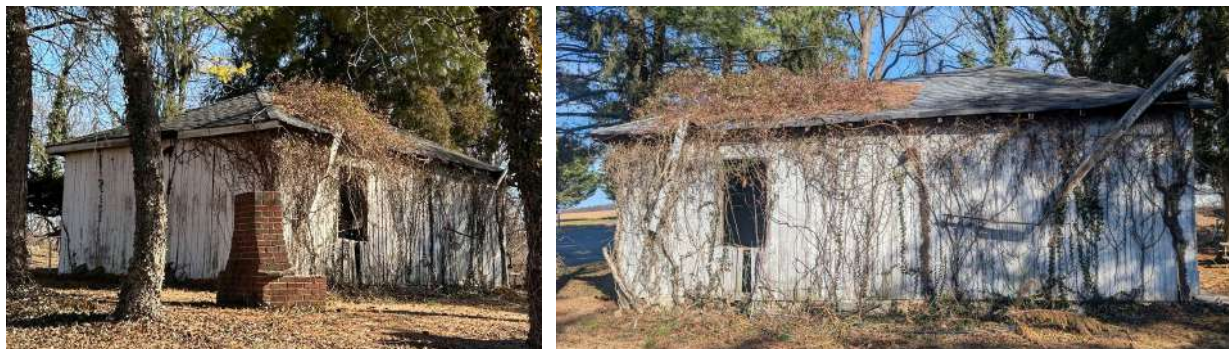
Figure 4: View of the northwest and southwest elevations of the existing garage (left) and southwest elevation (right).
