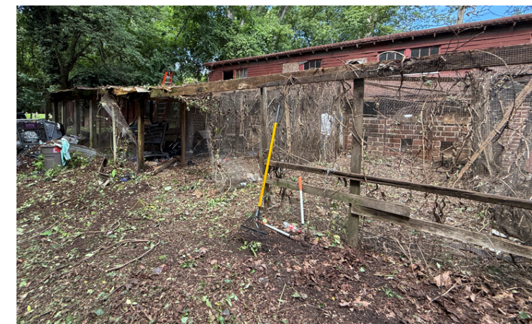
①⑪ Historic Kennel east facade (rear) with outdoor kennel runs visible in foreground
