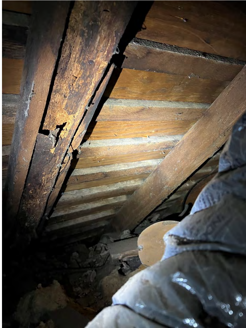
Photograph 25 – Typical severely deteriorated wood roof framing observed in attic space.
