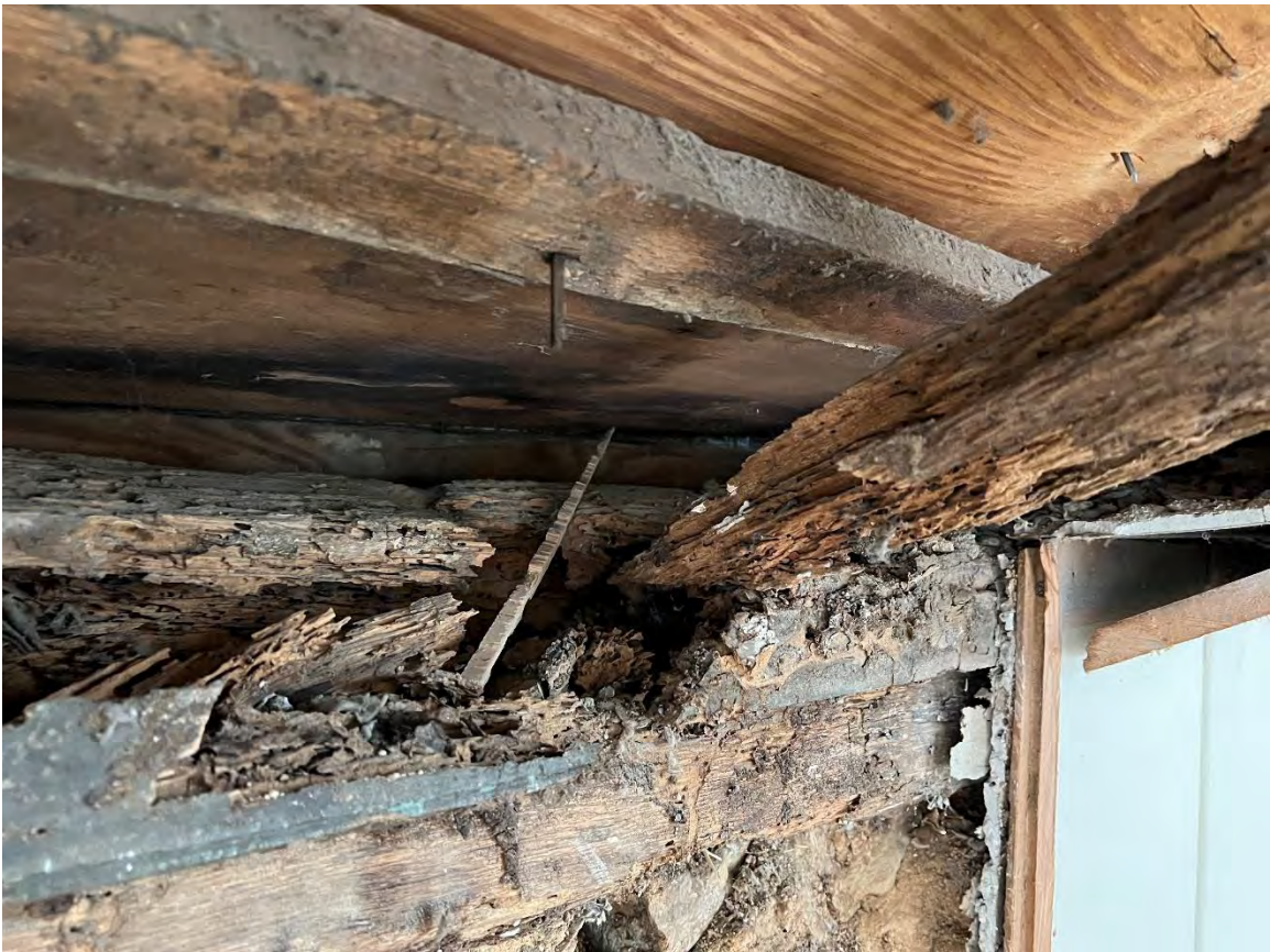
Photograph 22 – Typical severely deteriorated wood roof framing.
