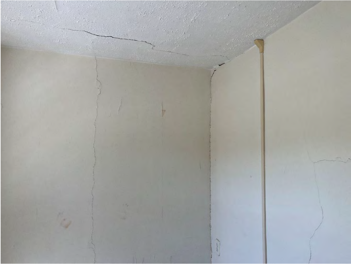
Photograph 17 – Typical cracks in interior wall/ceiling finishes.
