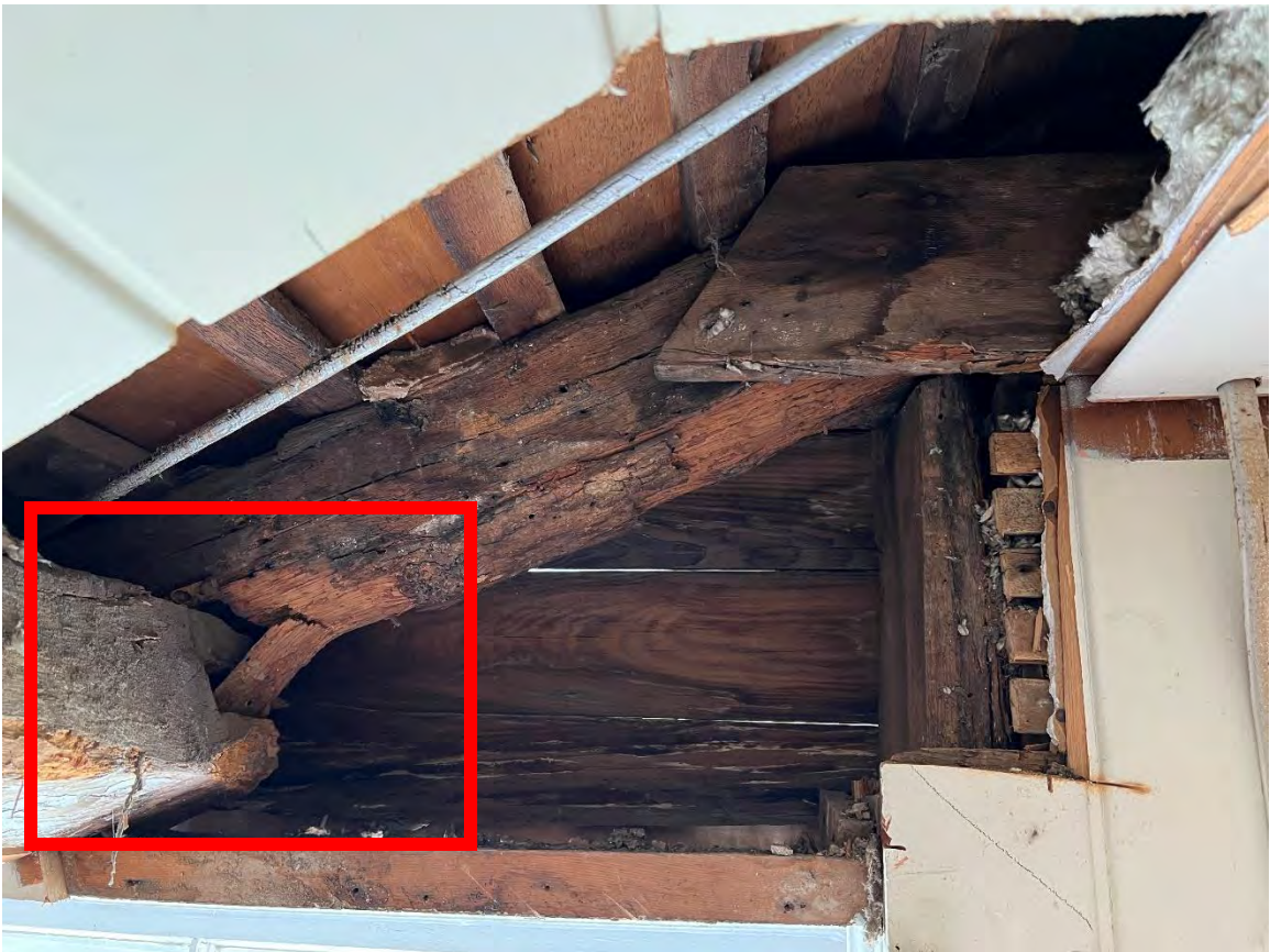
Photograph 24 – Failed connection between rafter and intermediate beam.
