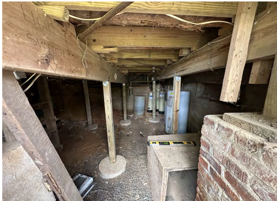
1. Basement Mechanical Space showing multiple layers of temporary supports and failing floor joists (photo by TEC, June 2025).
