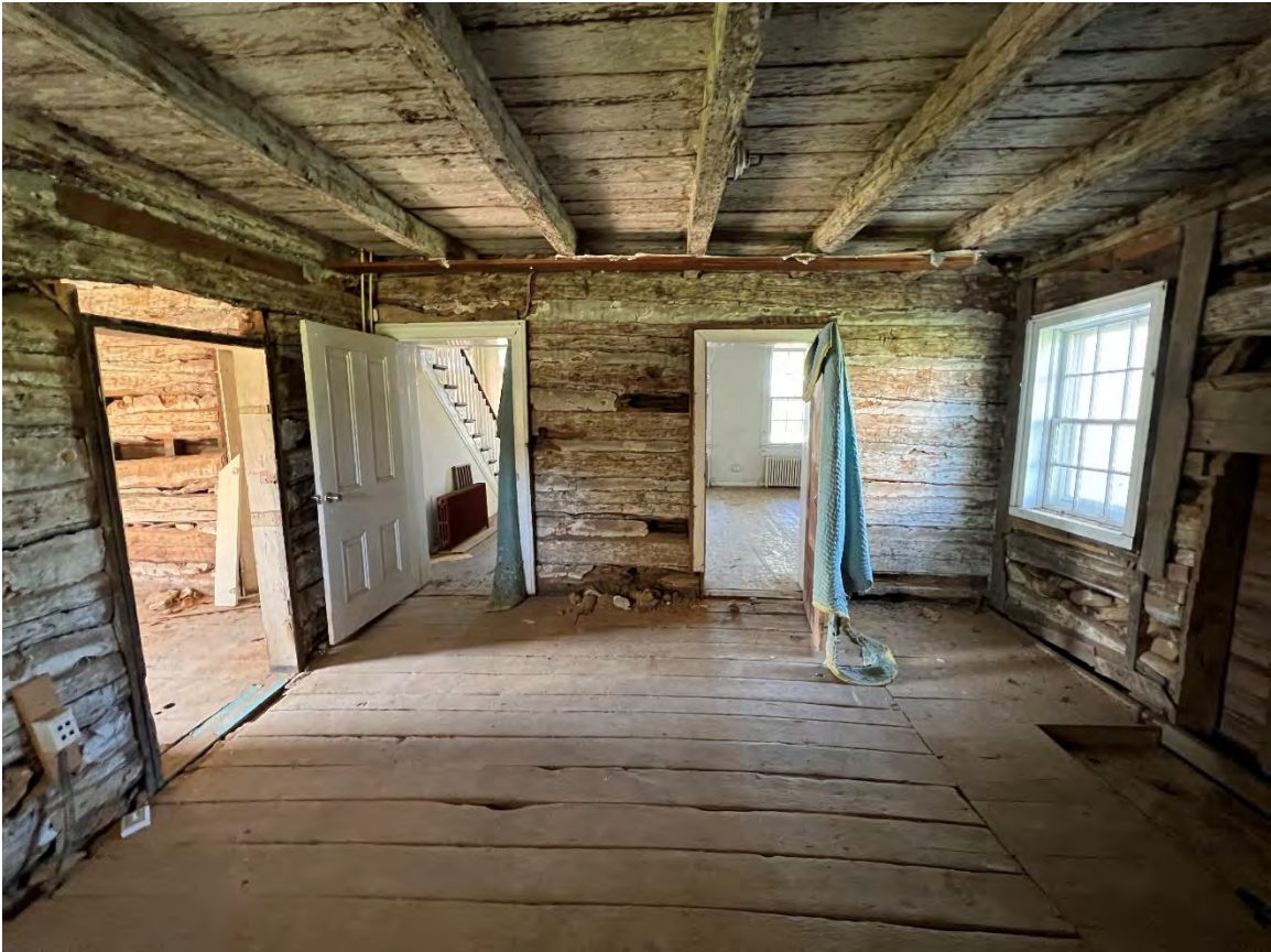
Photograph 14 – Large bow in floor in Room 1D.
