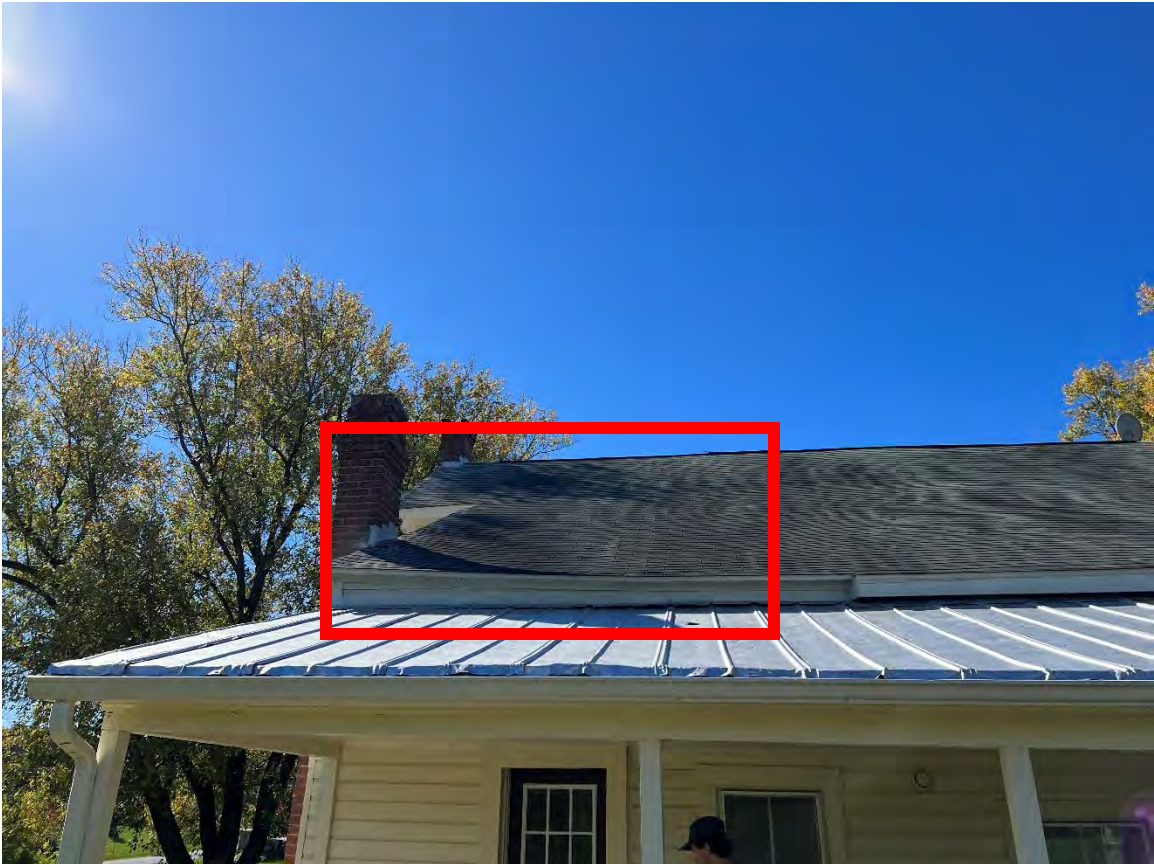
Photograph 20 – Typical sag in roof.
