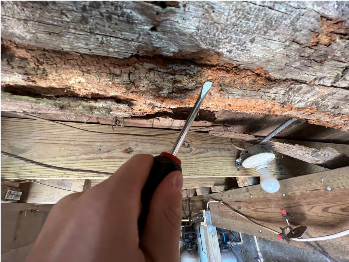
Photograph 4 – Typical poor condition of original log house first floor framing (logs).
