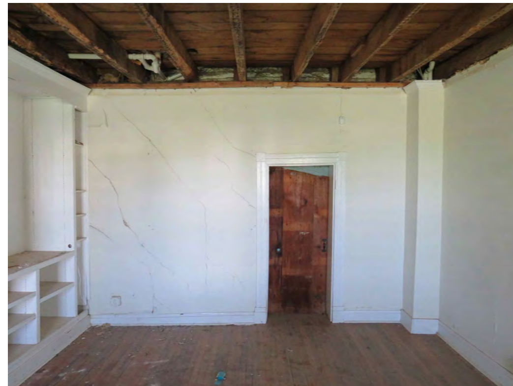
P ROOM 1A - REAR VIEW
