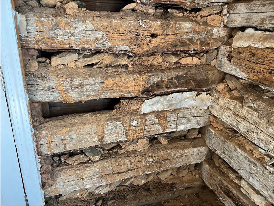
Photograph 11 – Typical poor condition of log walls within log house interior.
