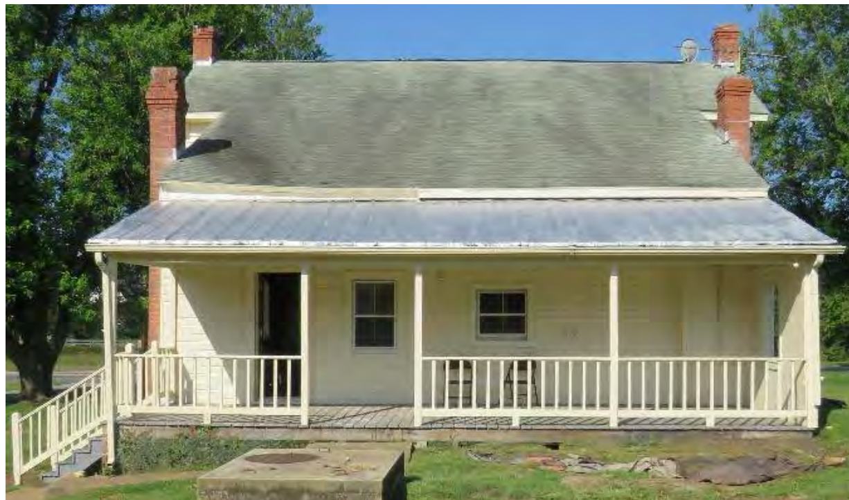
3. Rear Elevation, 2025. The rear of the house and porch would be completely rebuilt, but without the chimneys and the porch side wing wall. A shed dormer is proposed for the second floor to allow light and the required headroom for the master bedroom. Other openings on the first floor will be adjusted. (See other photos and drawings.)
