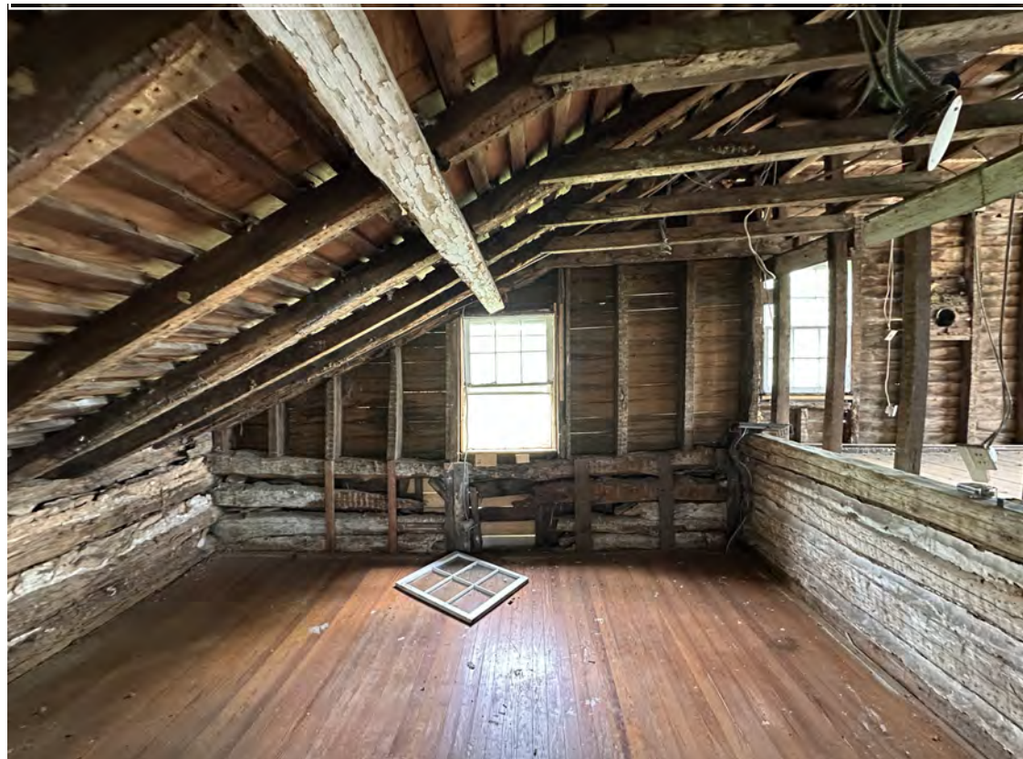
3. Primary roof beam rests unsupported on the window trim. Deteriorated log walls under the window and roof (photo by TEC, June 2025).
