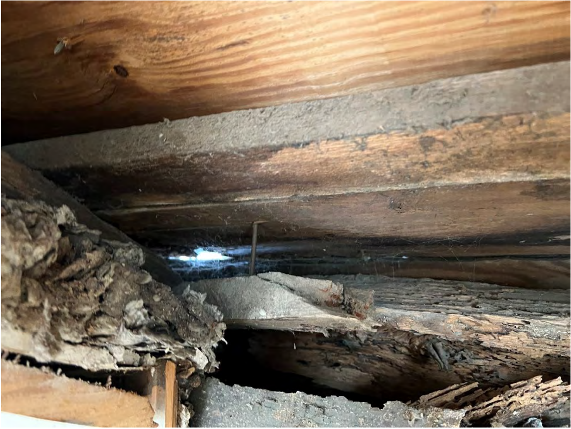
Photograph 23 – Typical severely deteriorated wood roof framing and daylight present.
