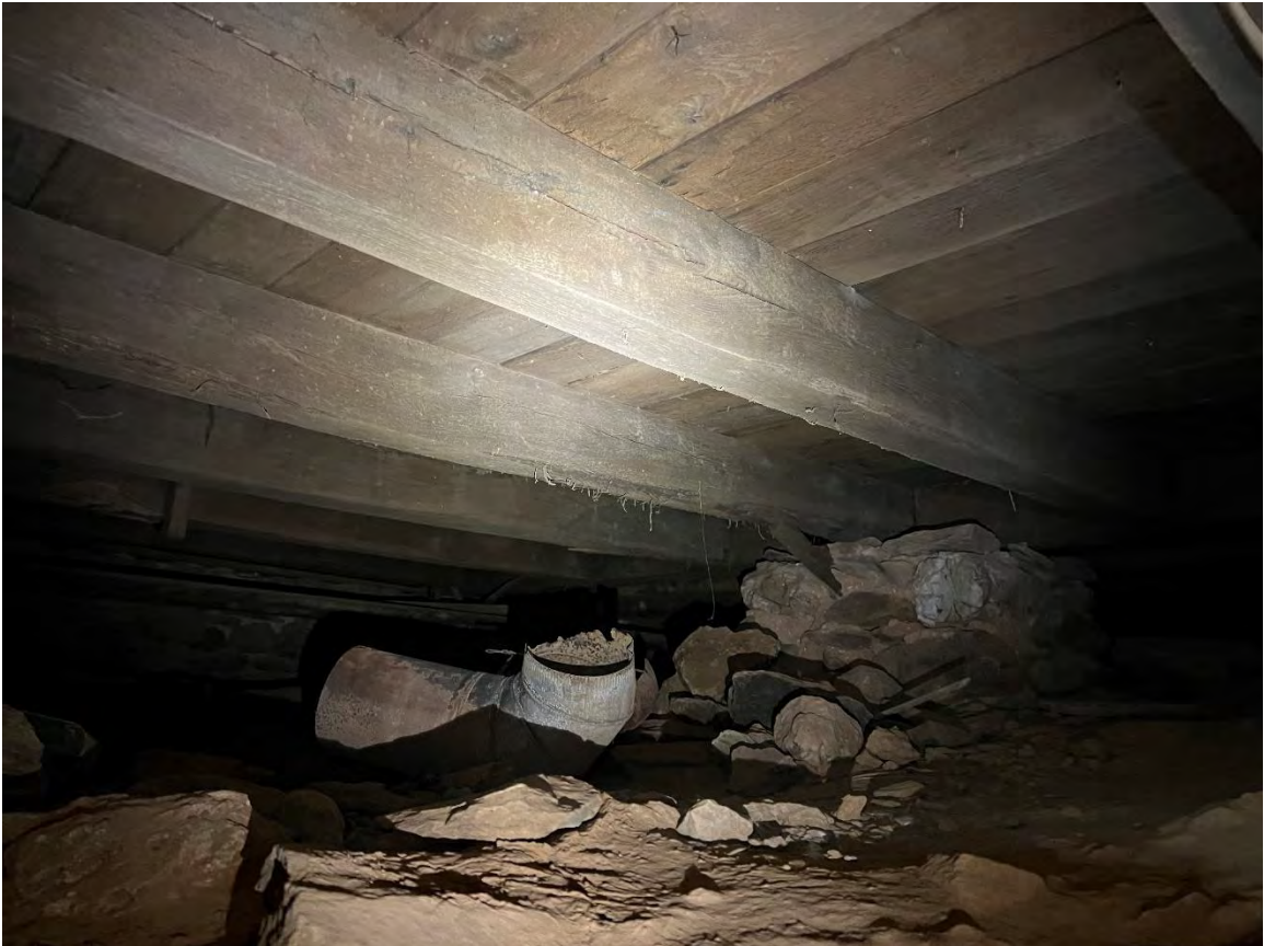
Photograph 8 – Typical timbers supporting first floor of Rooms 1A and 1B of addition.
