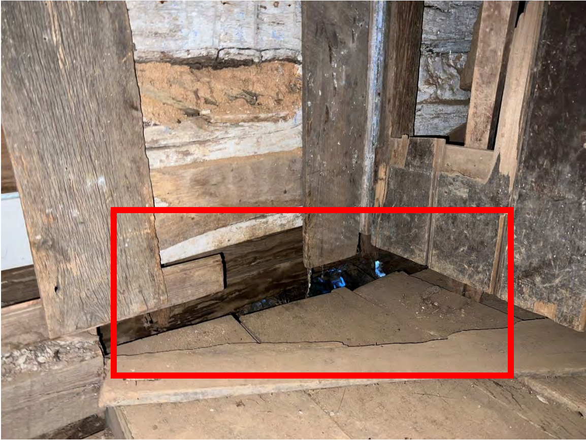
Photograph 13 – Deteriorated wood wall/floor framing at north end of Room 1D.
