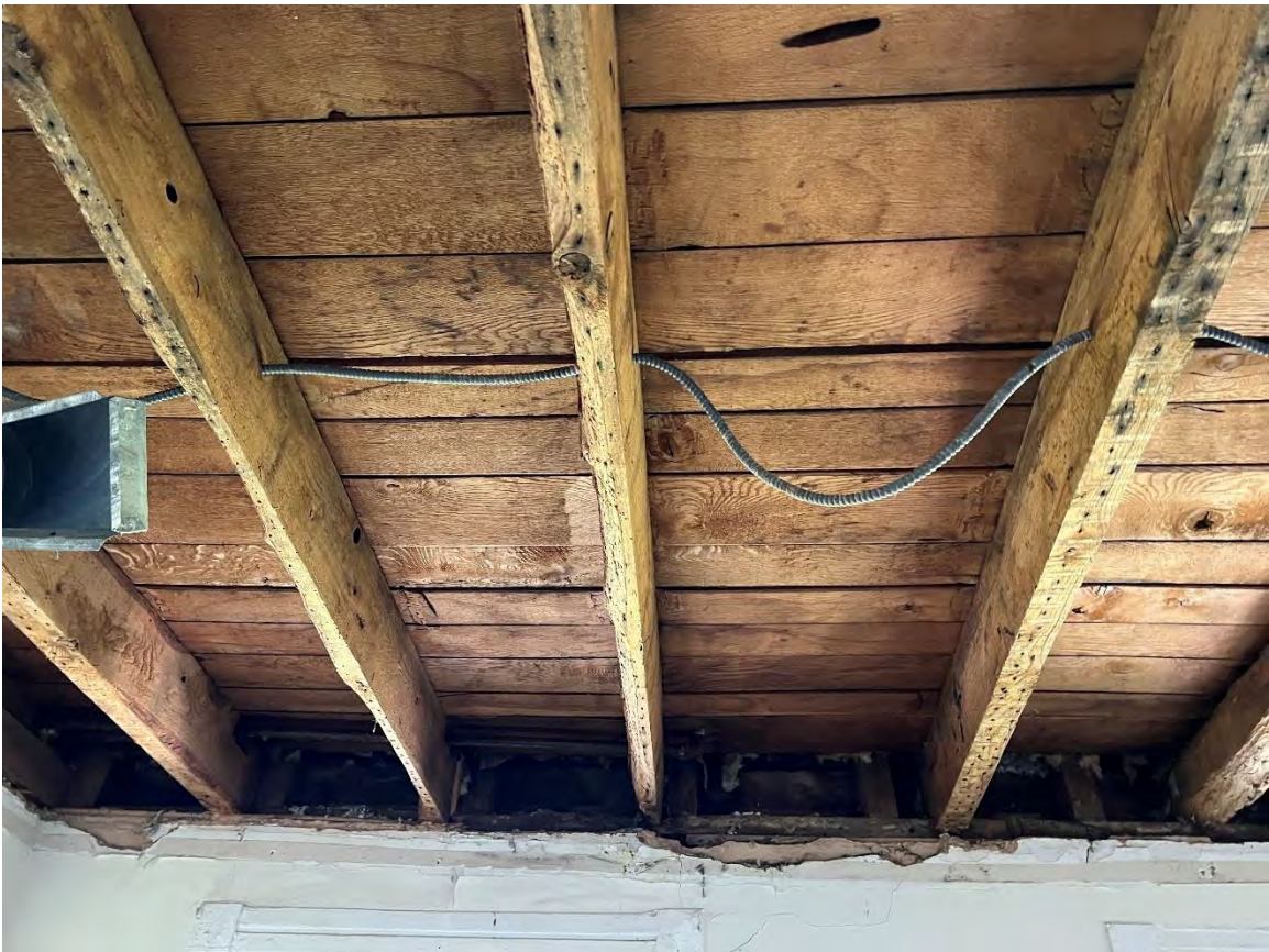
Photograph 18 - The floor joists supporting the upper levels were inconsistently sized with the widths ranging from four (4) inches wide to as narrow as one (1) inch wide.
