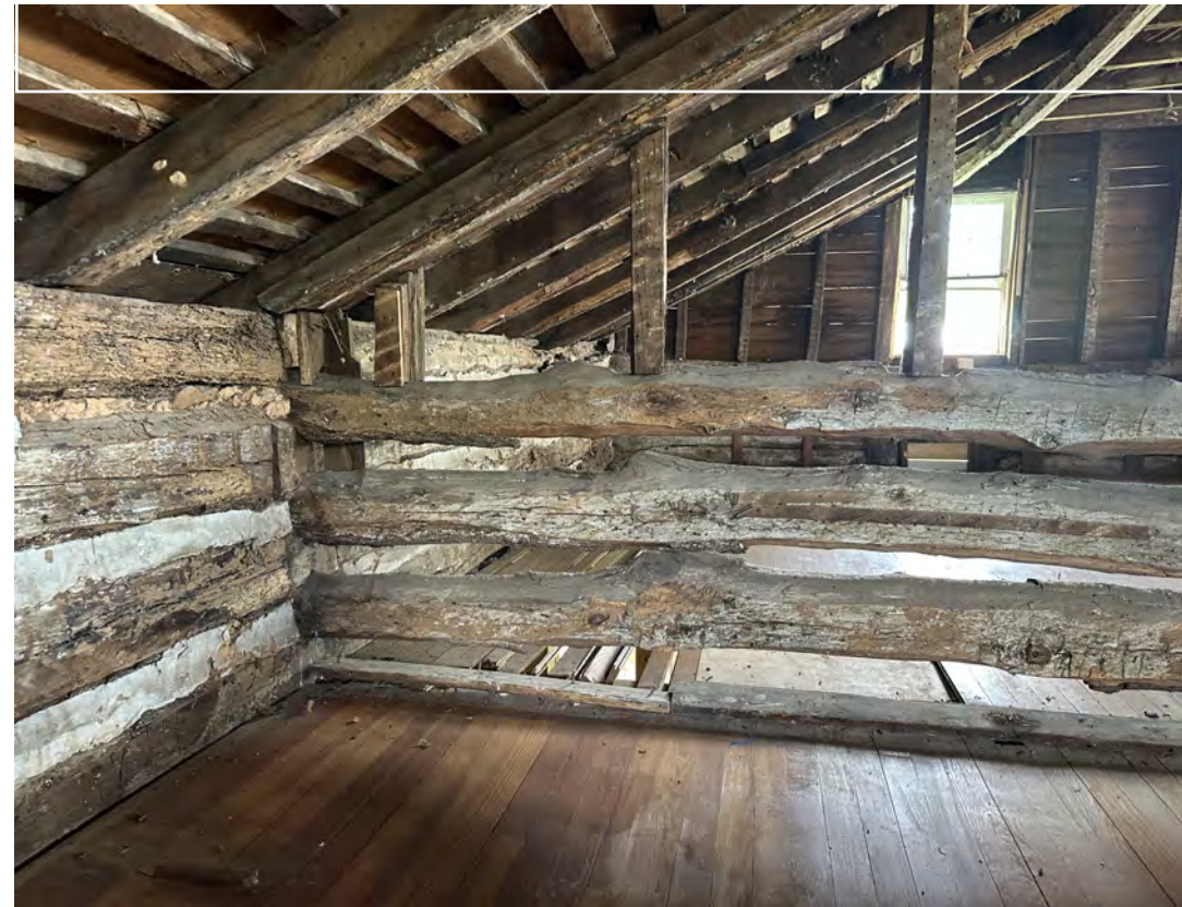
4. Failing log walls entirely ineffective in supporting the roof structure (photo by TEC, June 2025).
