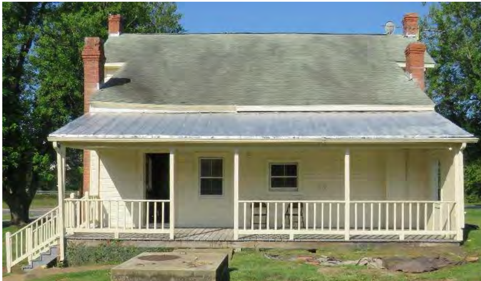
1. Rear elevation showing roof sagging and current window and door openings. This portion of the house and porch will be completely rebuilt except for the rear chimneys and porch wing wall. Window and door openings will be slightly modified to accommodate the new floor plan, see photos 3 & 4 below.
