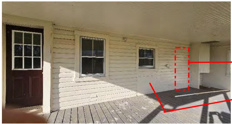
3. Rear elevation view from the back porch showing existing window and door openings.
