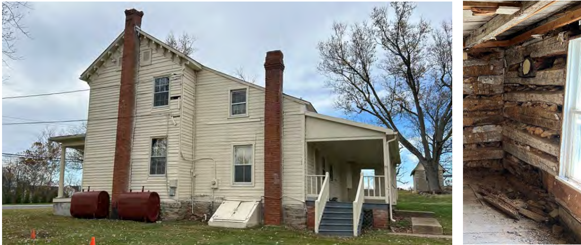
Figure 3: Existing southeast elevation (left) and interior view of the vent pipe and first-floor 2-over-2 window (right).
