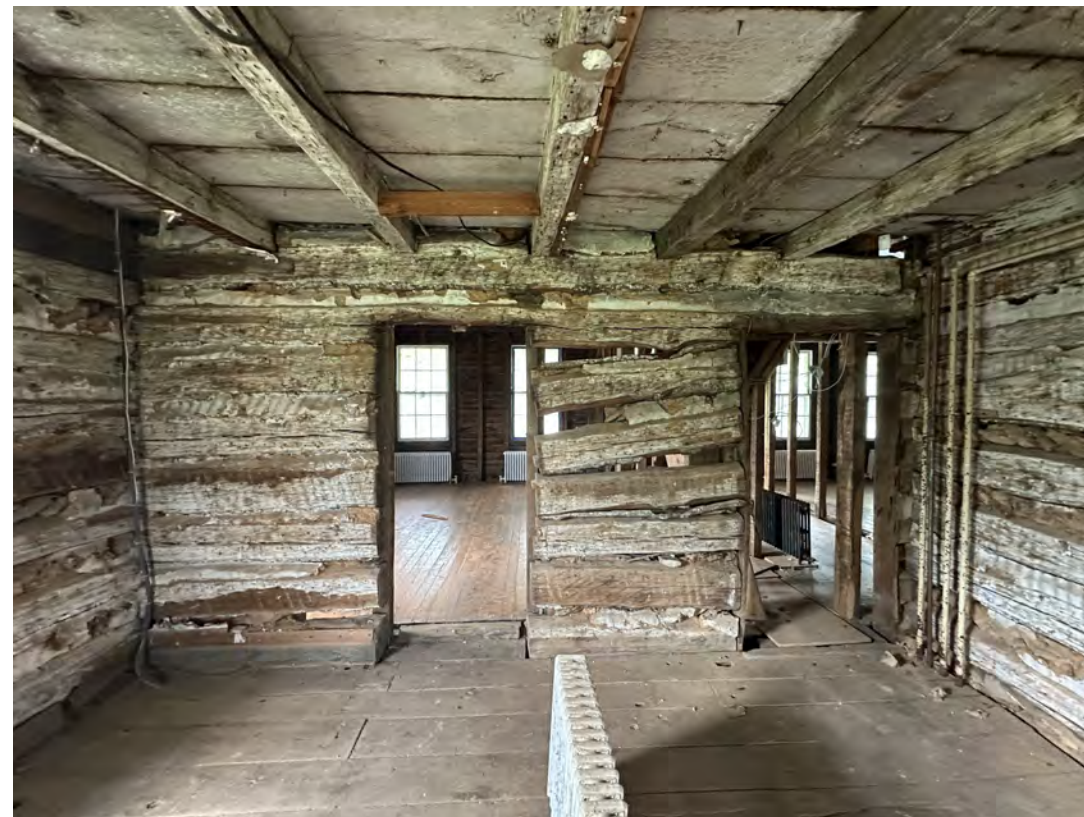
2. Deteriorated log walls failing to provide support for the floor above (photo by TEC, June 2025).
