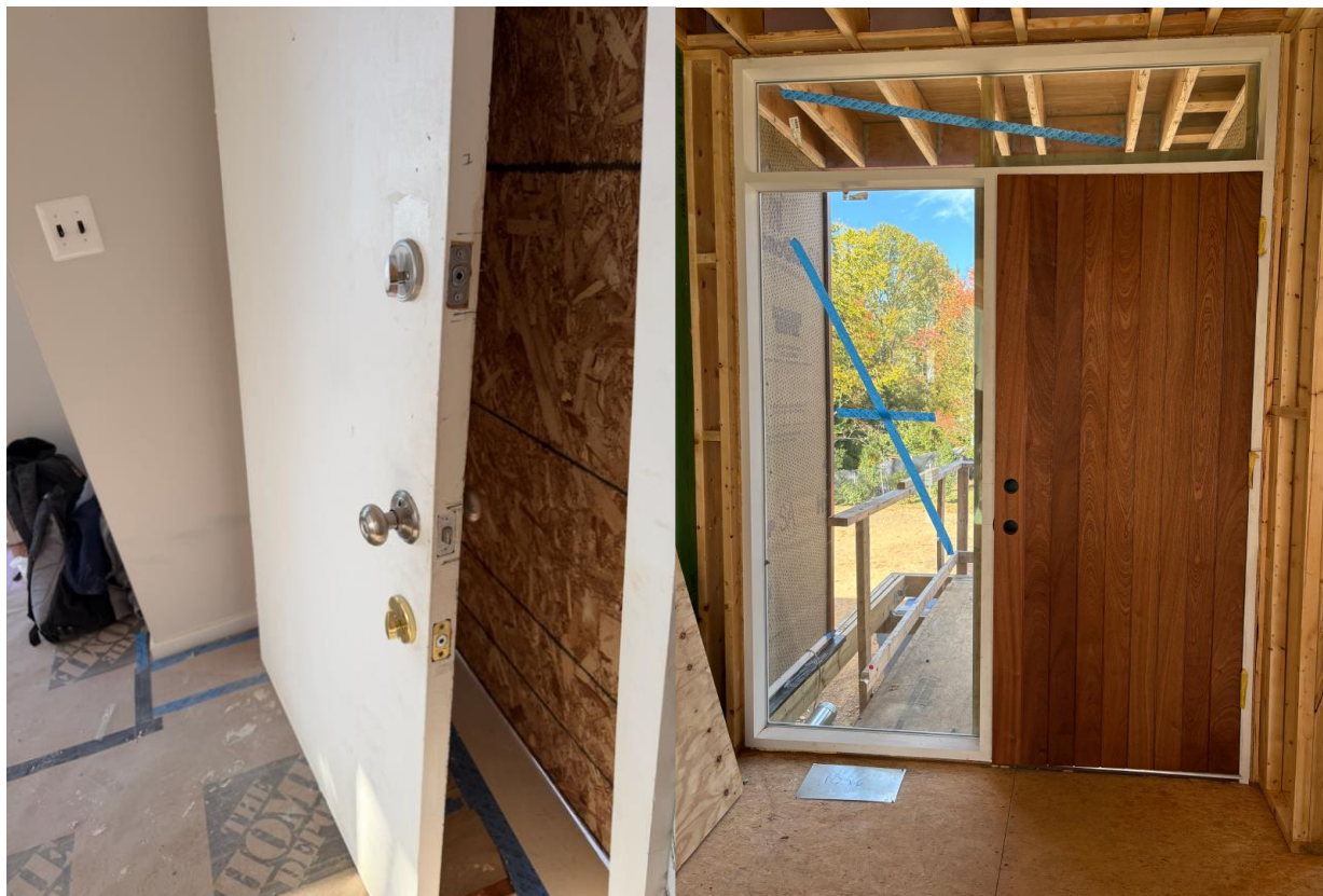
Figure 3: Existing door showing damage (left) and precedent image of the proposed door (right)._
