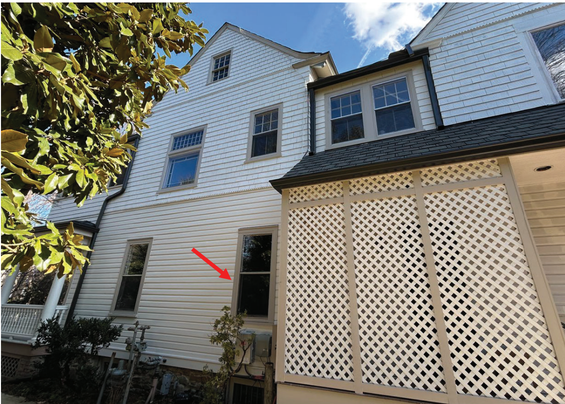
Figure 10: Portion of the existing west side elevation (January 2026, Historic Preservation Division). A red arrow points to the window proposed to be replaced with tempered, frosted glass.
