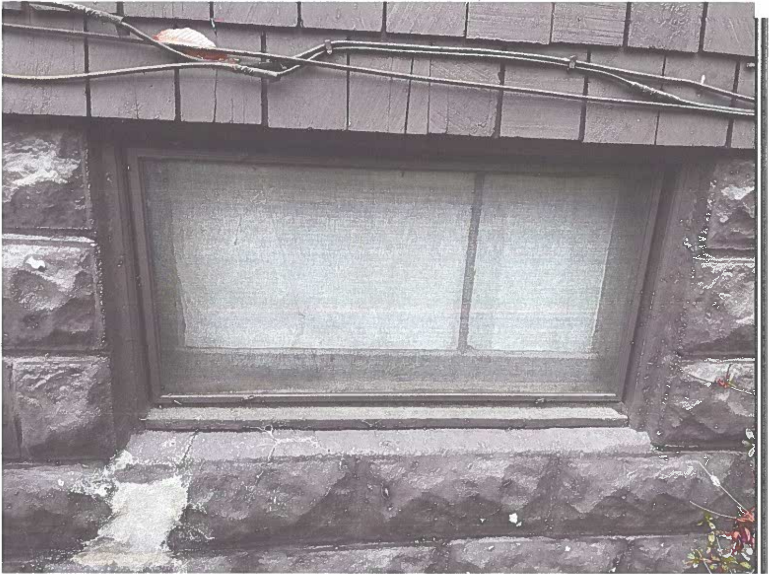
NORTH SIDE WINDOW MISSING 1 MUNTIN
