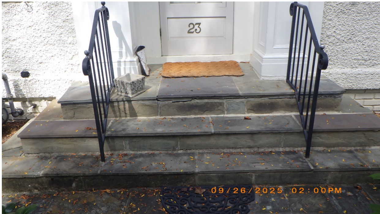
Figure 2. Existing front portico/step to be replaced.
