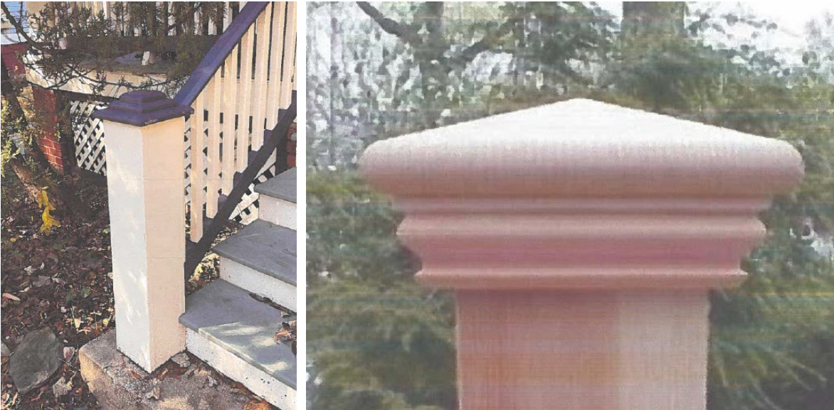
Figure 5: Existing newel post and railing detail, left; and proposed newel post cap, right.
