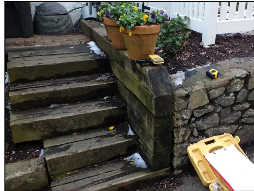
Existing Timber Stairs to Be Removed and Stone Wall to Remain (November, 2025)
