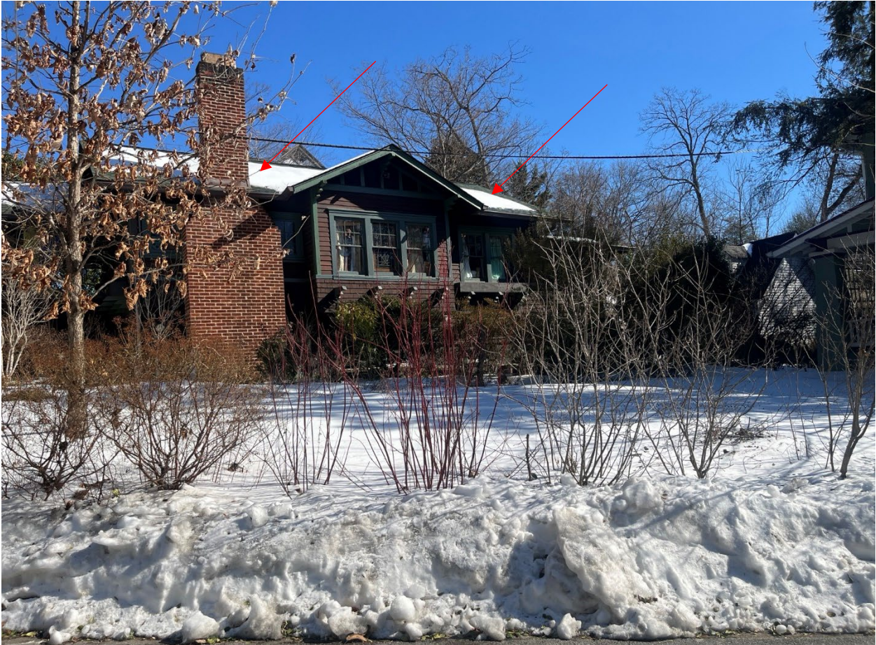
Figure 8: View of roof from right-of-way. The location of panels is notated with a red arrow.
