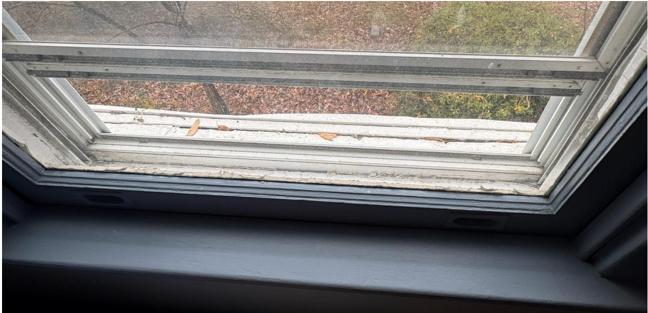
Figure 3: Detail of a gap between the truncated sill and aluminum siding.
