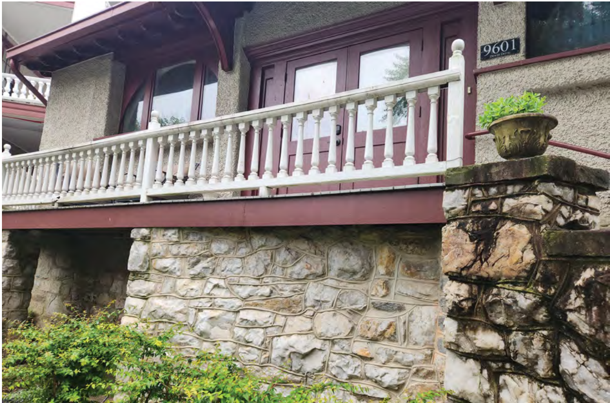
Figure 9: Front porch railings to be repaired.
