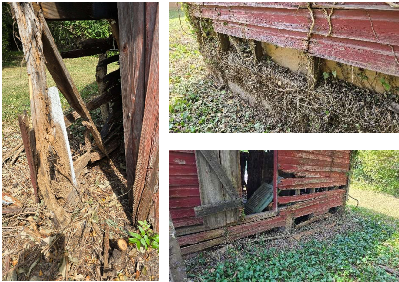
Figure 2 – Rotten wood at the base of the walls
