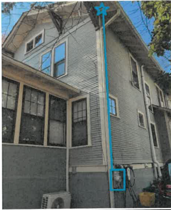
Utility Meter after Installation
