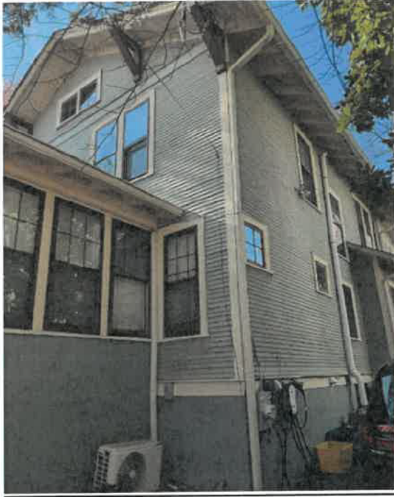
Utility Meter before Installation
