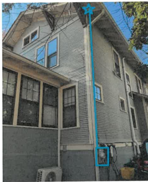
Utility Meter after Installation
