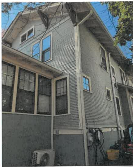
Utility Meter before Installation
