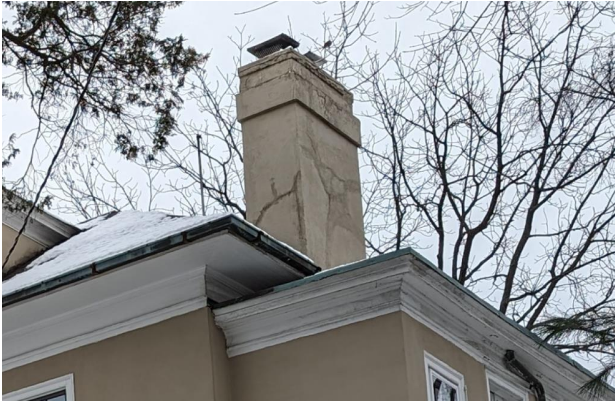
Figure 2: Photo of the chimney showing visible cracks and previous repairs.
