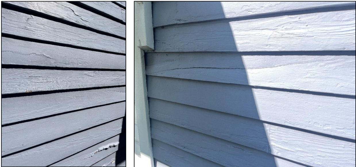
Figure 6: Details of some of the issues with the siding, including peeling paint and cracking, on the right side/south elevation.
