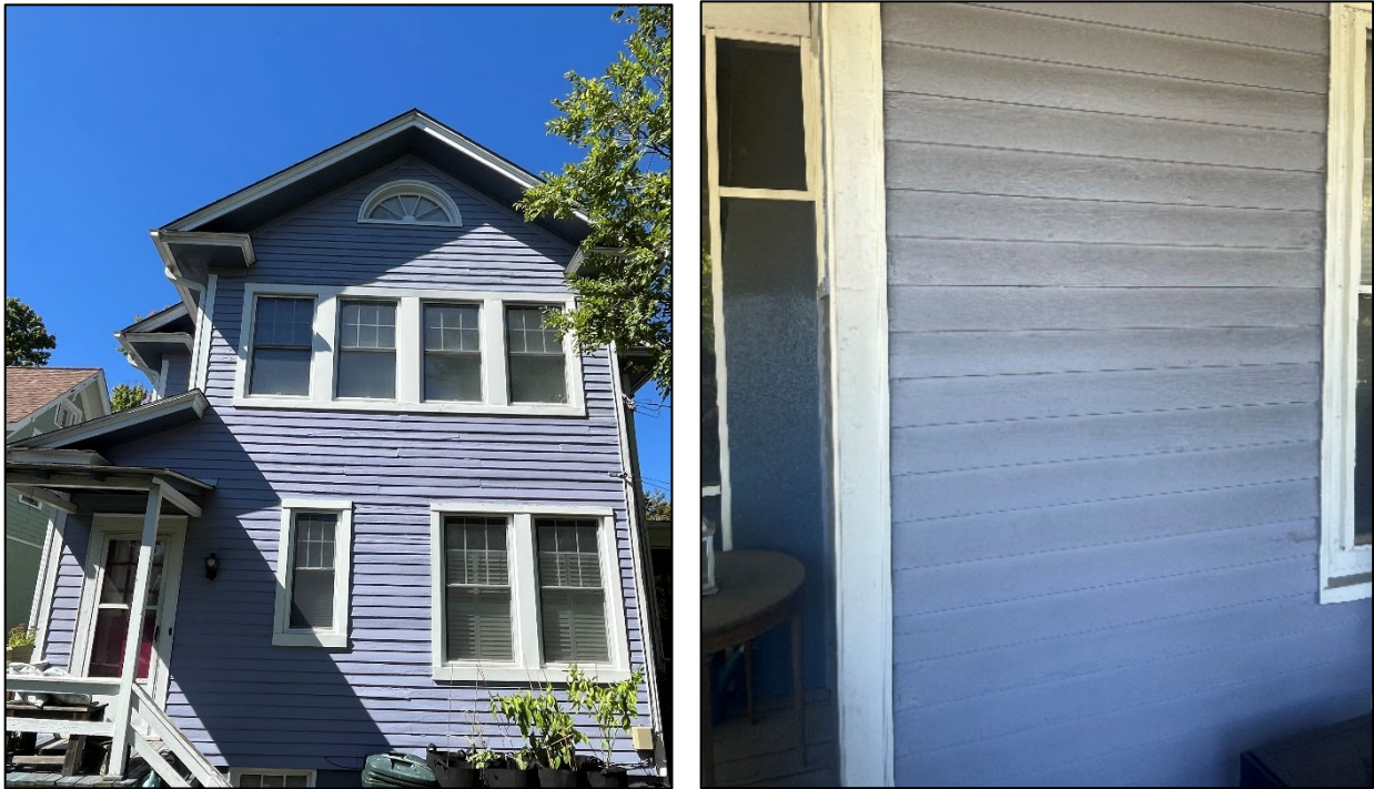
Figure 7: Details of the condition of the boards. Note that the boards on the rear/north elevation (left) show some signs of warping, while the boards on the front porch appear to be in good condition (right).
