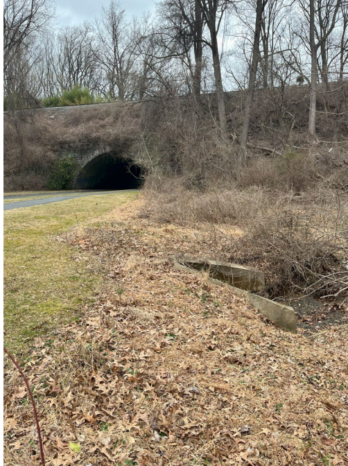
Photograph 1: Beach Dr roadway embankment, slope, and existing culvert. facing the B&O Viaduct
