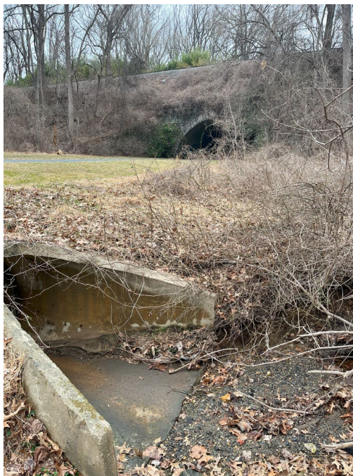
Photograph 2: Existing culvert under Beach Dr. and drainage way facing the B&O Viaduct
