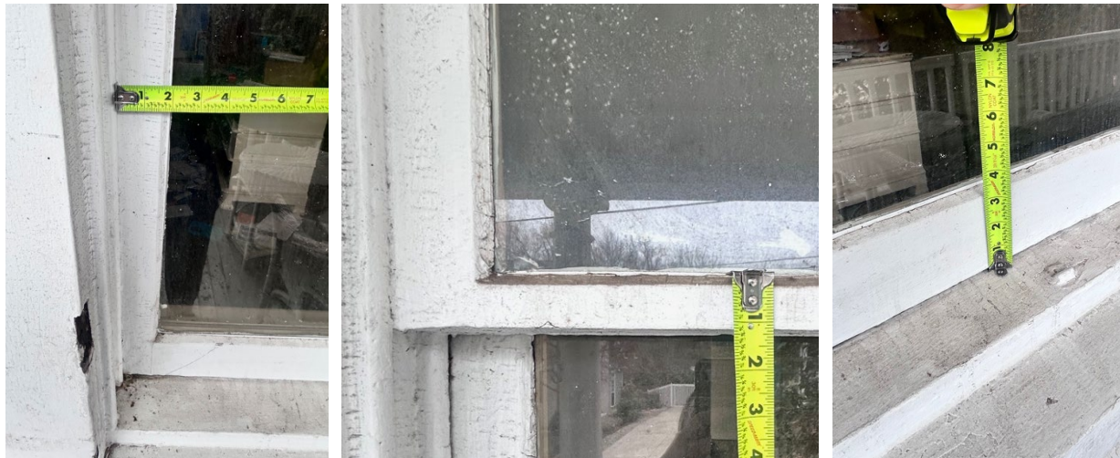
Figure 13: Select dimensions of existing first-floor windows, left to right: side rail, meeting rail, and bottom rail (Historic Preservation Office, March 2025).
