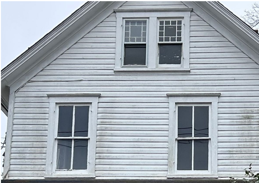
Figure 15: Front elevation photograph showing the existing Queen Anne attic windows and 2-over-2 second-floor windows, as well as some of the existing shutter hardware.
