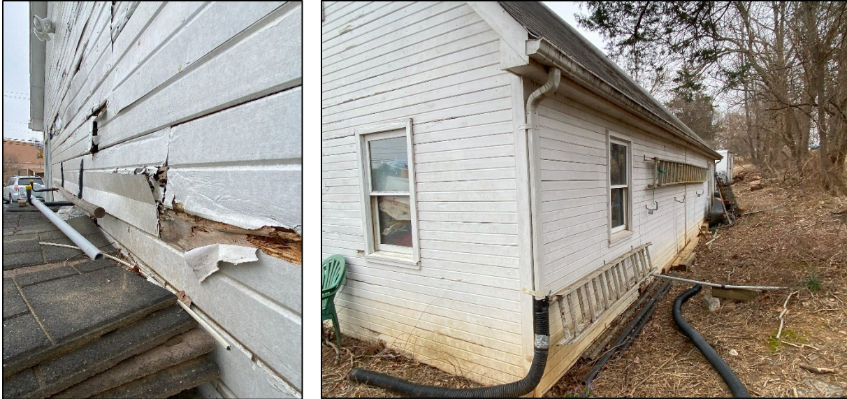
Figure 4: Detail of the wood condition on the west elevation (left) and view of north elevation (right). Both photos are courtesy of Montgomery County Planning, 2
