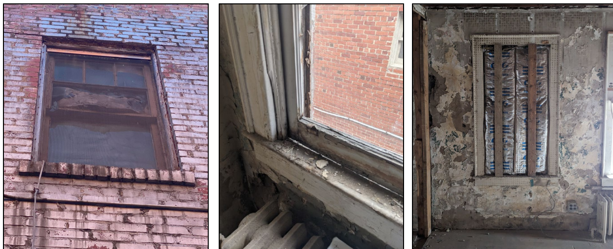
Figure 10: Condition of exterior windows (left; Montgomery County Planning Staff, 2025; center and right, Applicant, 2025). Three windows are boarded up from the inside, and their specific condition has only been assessed from the street level on the exterior.
