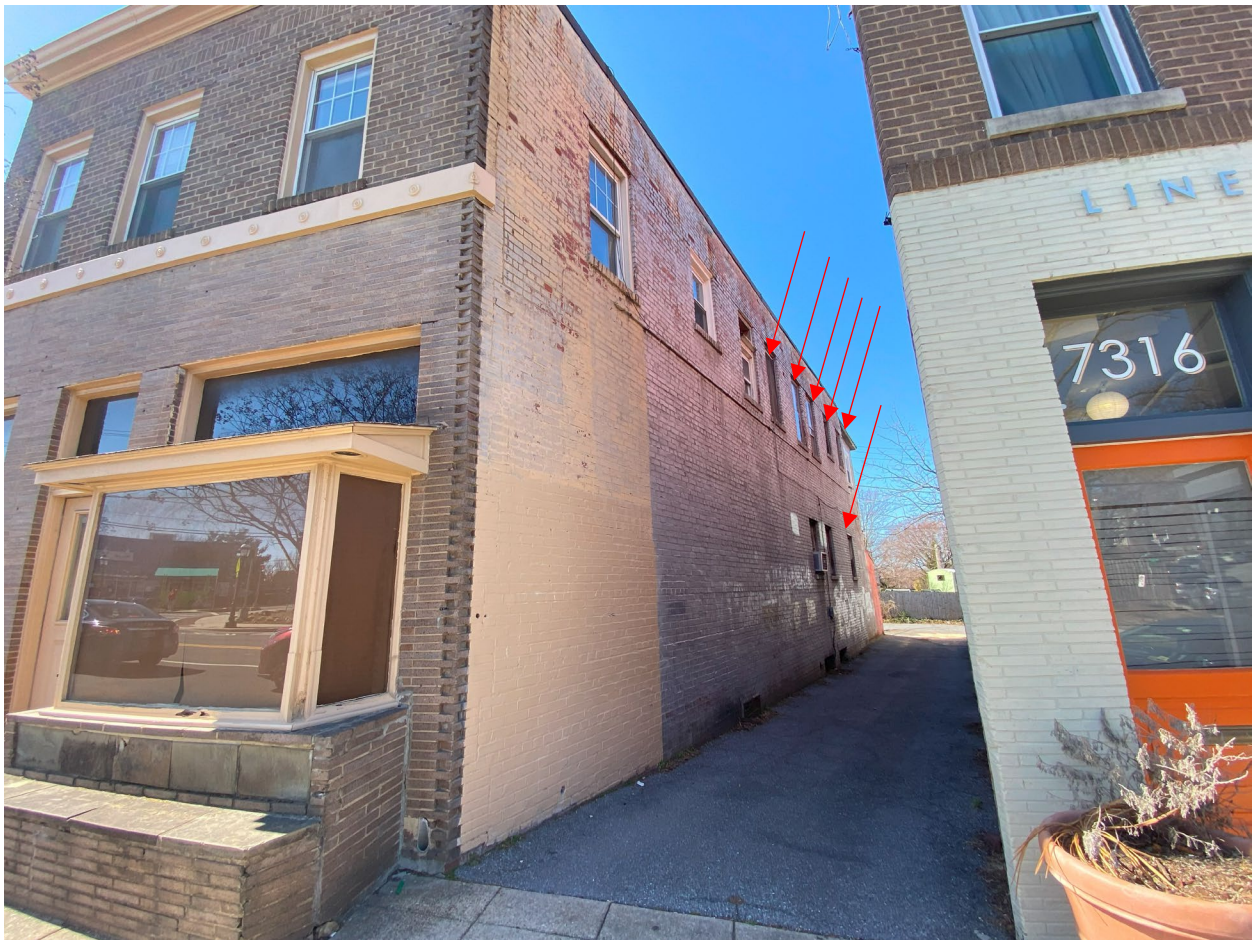
Figure 11: View of the side elevation, with red arrows noting the location of wood windows (Montgomery County Planning, 2025).
