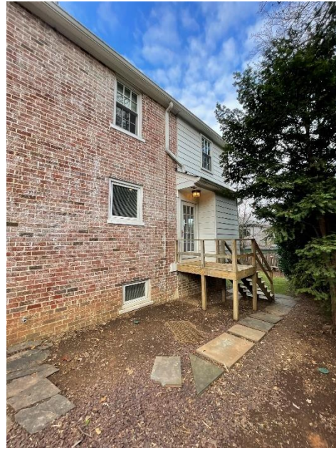
Existing East side of the House looking towards the rear and n seeing the existing side addition
