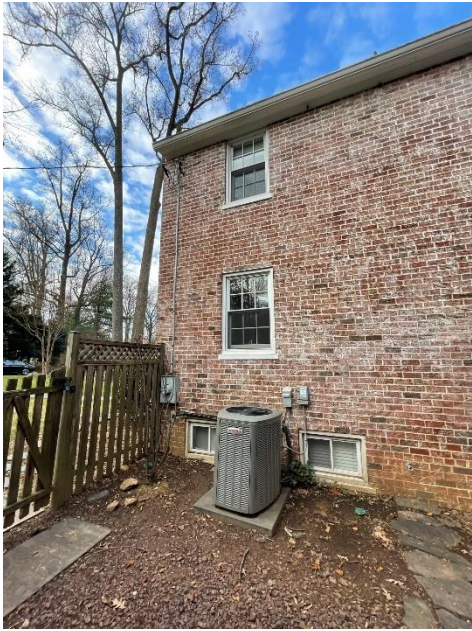
Existing East side of the House looking towards the street (Fence and A/C unit to remain)
