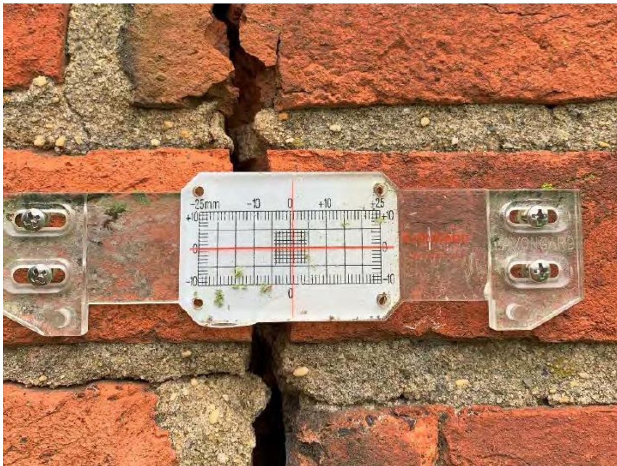
Figure 4: One of the crack monitors shows the crack has spread by approximately 1mm (one millimeter).
