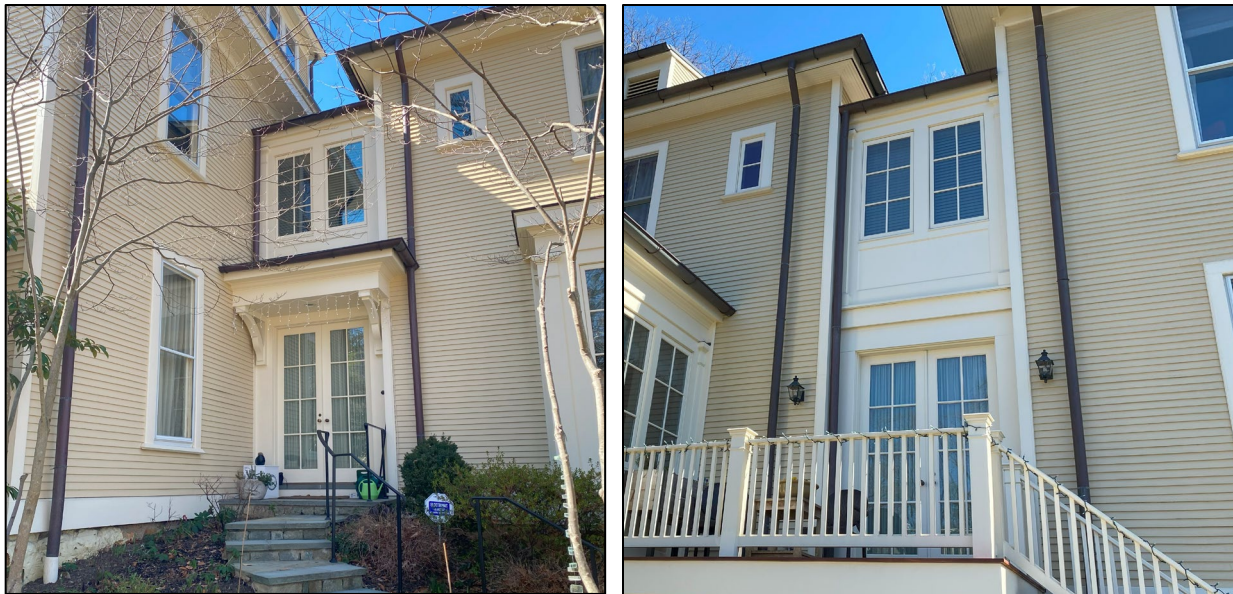
Figure 6: The left/east awning awning (left) and the right/west awning (right) of the subject property (Montgomery County Planning, 2025).
