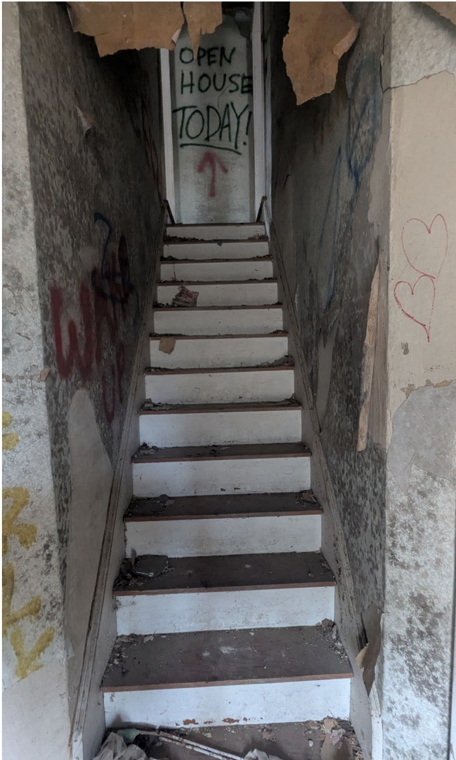
Figure 35: Conditions of interior staircase, Montgomery Planning, 2025.
