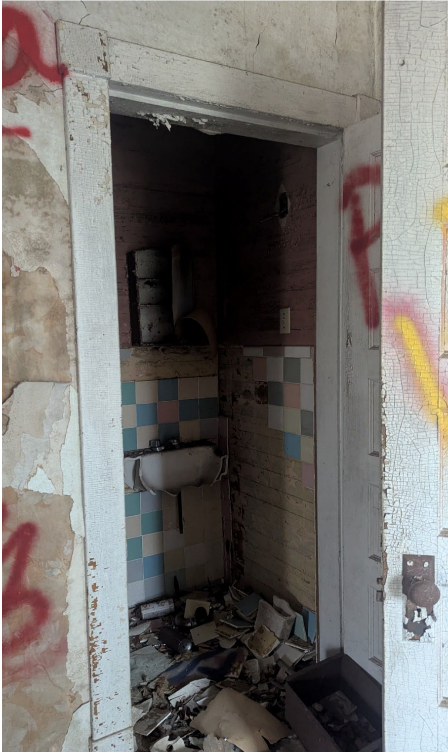
Figure 33: Conditions of bathroom, Montgomery Planning, 2025.
