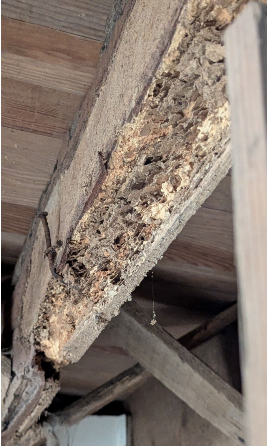
Figure 30: Damage to joists under house, Montgomery Planning, 2025.
