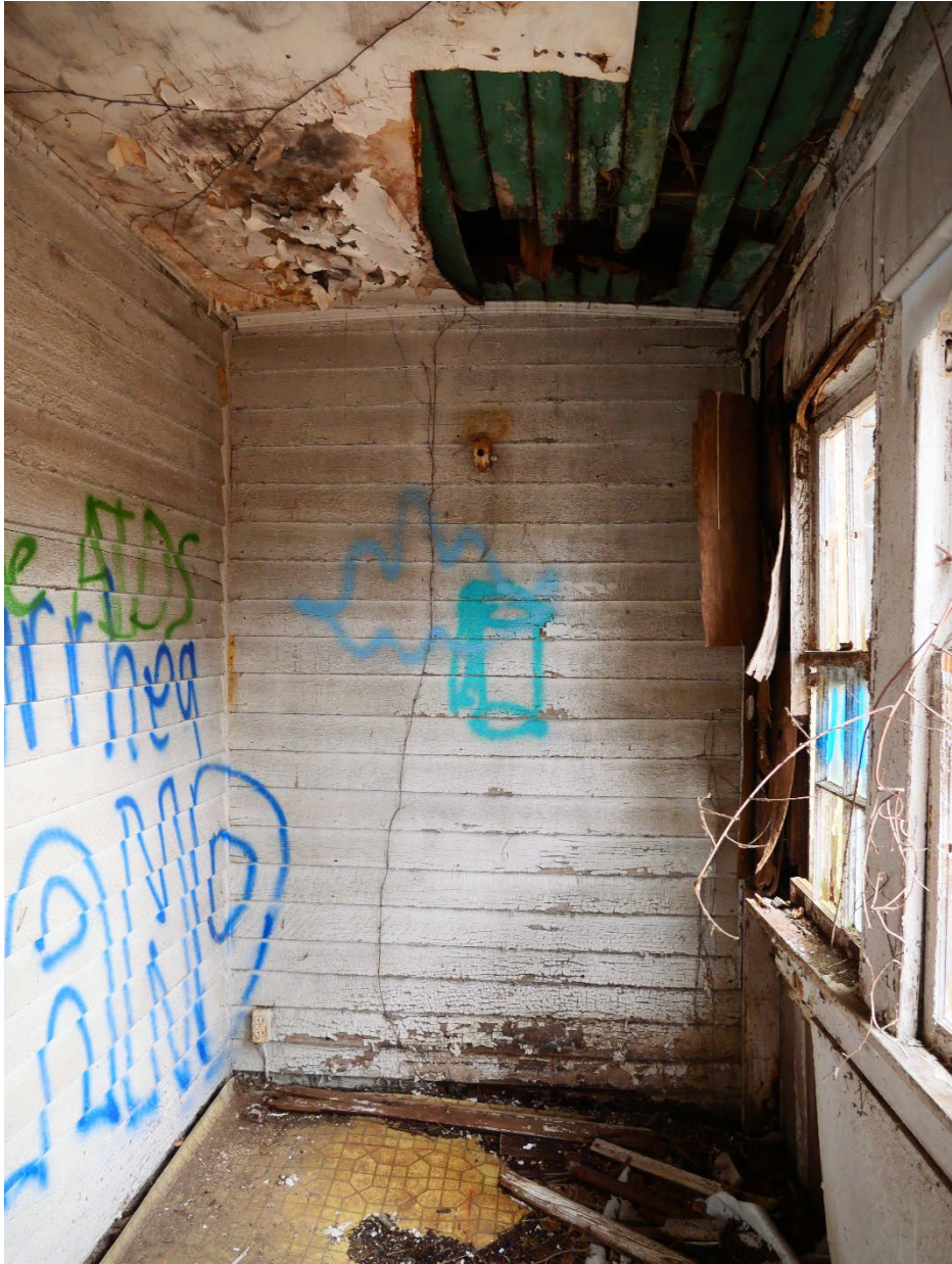
Figure 31: Conditions inside enclosed porch, Montgomery Planning, 2025.
