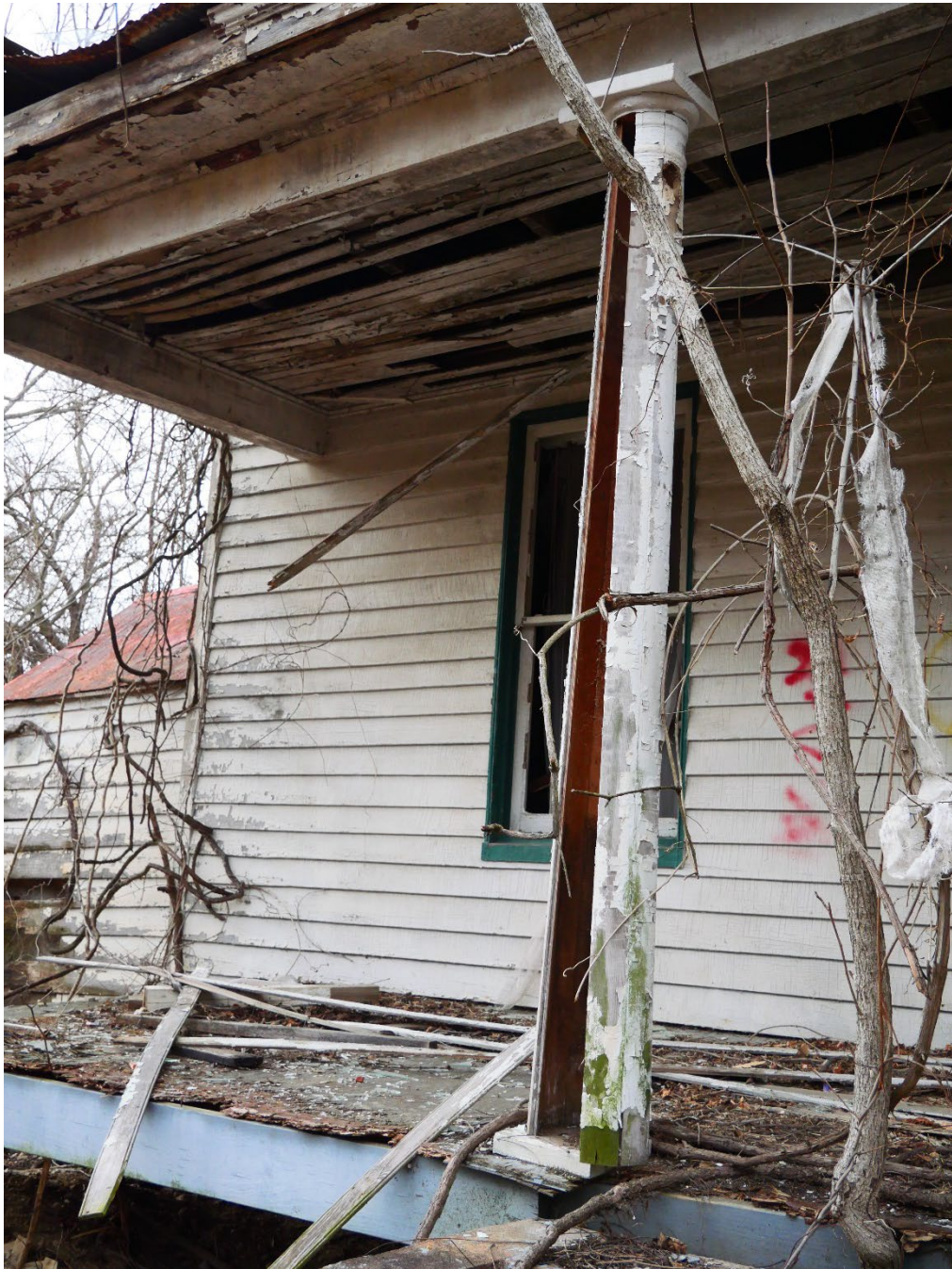
Figure 25: Close up of conditions of porch roof, Montgomery Planning, 2025.
