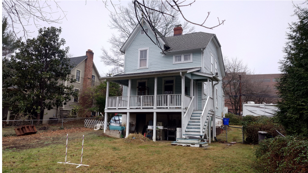
Rear Photo Wood porch to be removed
