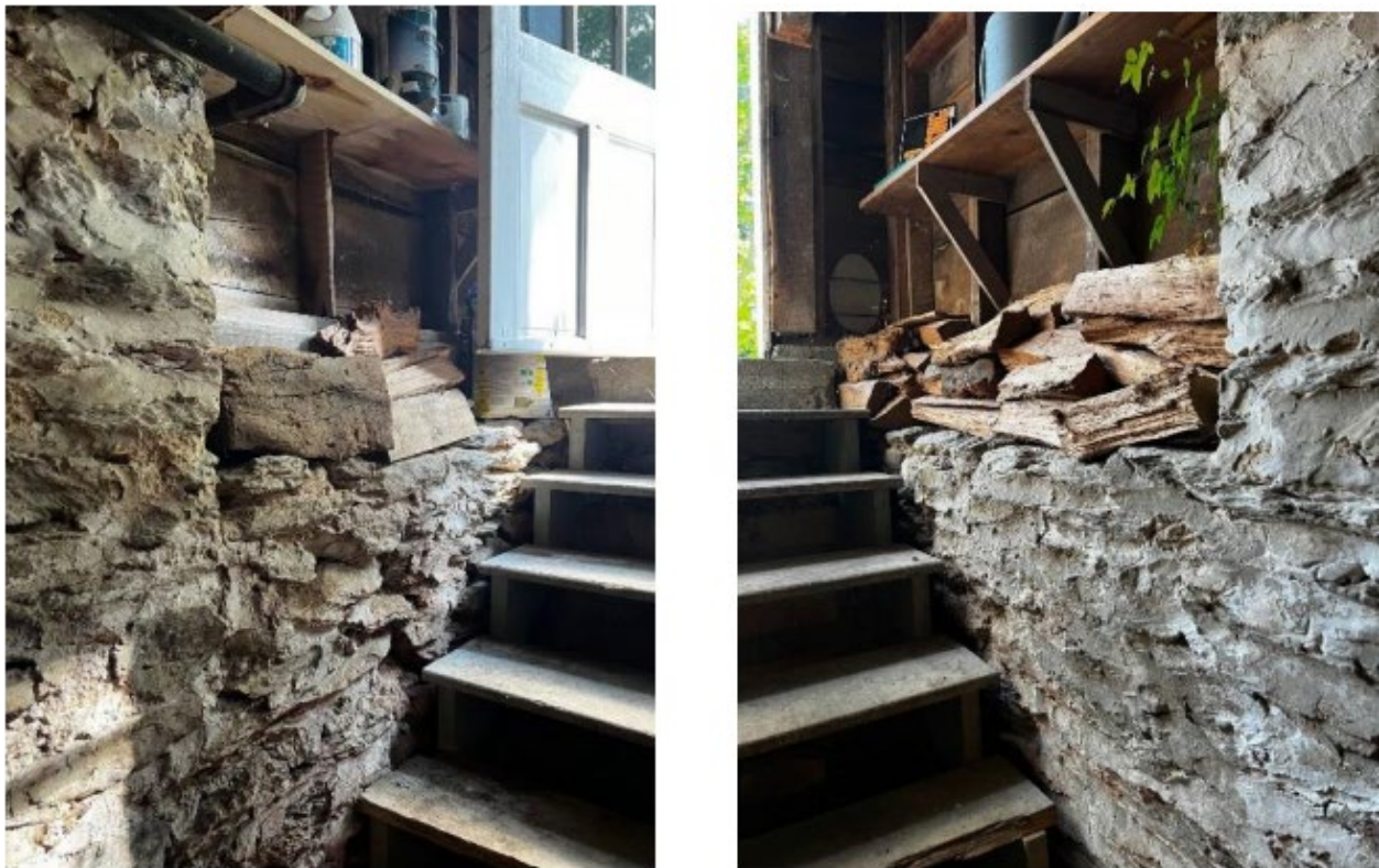
Figure 9: Supplemental photographs of the interior of the vestibule and walls along the cellar steps.
