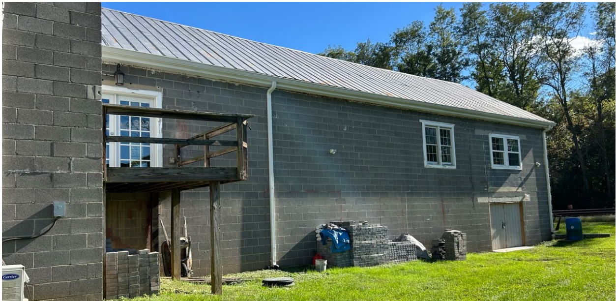
Figure 16: West elevation of the rear CMU addition, October 2024 (Historic Preservation Office). Recent window alterations have been undertaken, and additional alterations are proposed.
