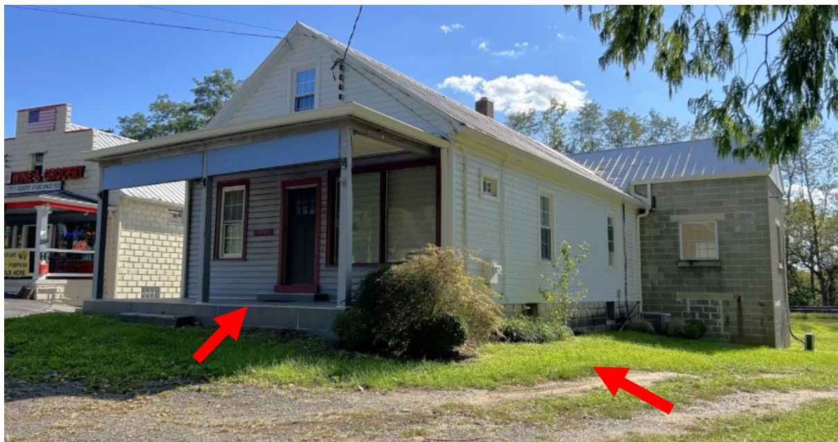
Figure 5: Front (north) and west side elevations, October 2024 (Historic Preservation Office). The red arrows points to the location of the proposed porch alterations and ADA ramp.
