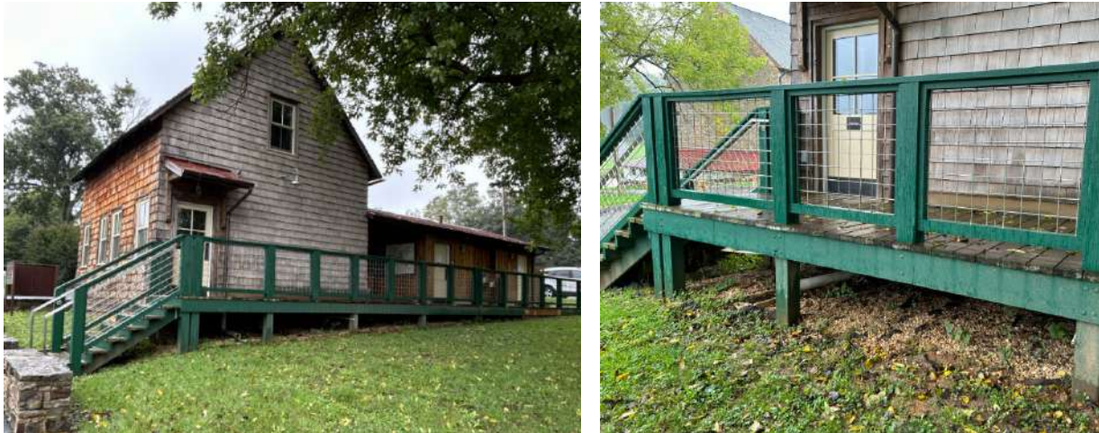
Figure 15: Example of mesh railing to be used on raised ramp (Work Item 8).
