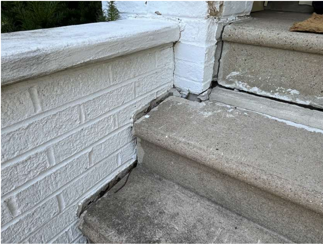
Detail: 7017 SYCAMORE AVE. CONCRETE STEPS
