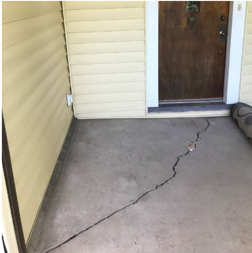
Detail: 7017 SYCAMORE AVE. CRACKED PORCH SLAB
