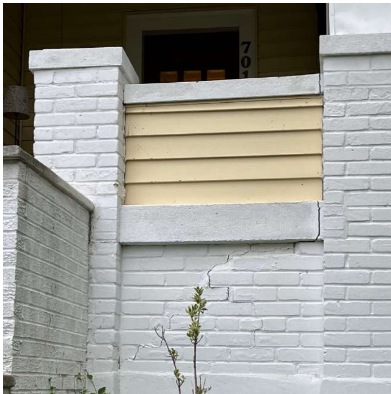
Detail: 7017 SYCAMORE AVE. PORCH FOUNDATION CRACKS
