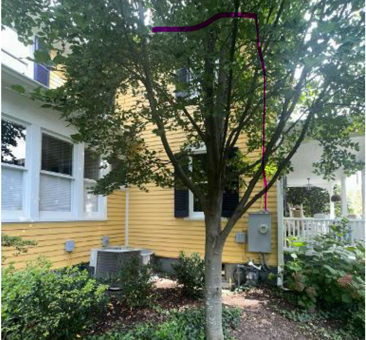
Utility Meter after install. This is the only picture I have. The tree is in the way of the view of how the conduit to be run up through the attic to the array on the roof.
