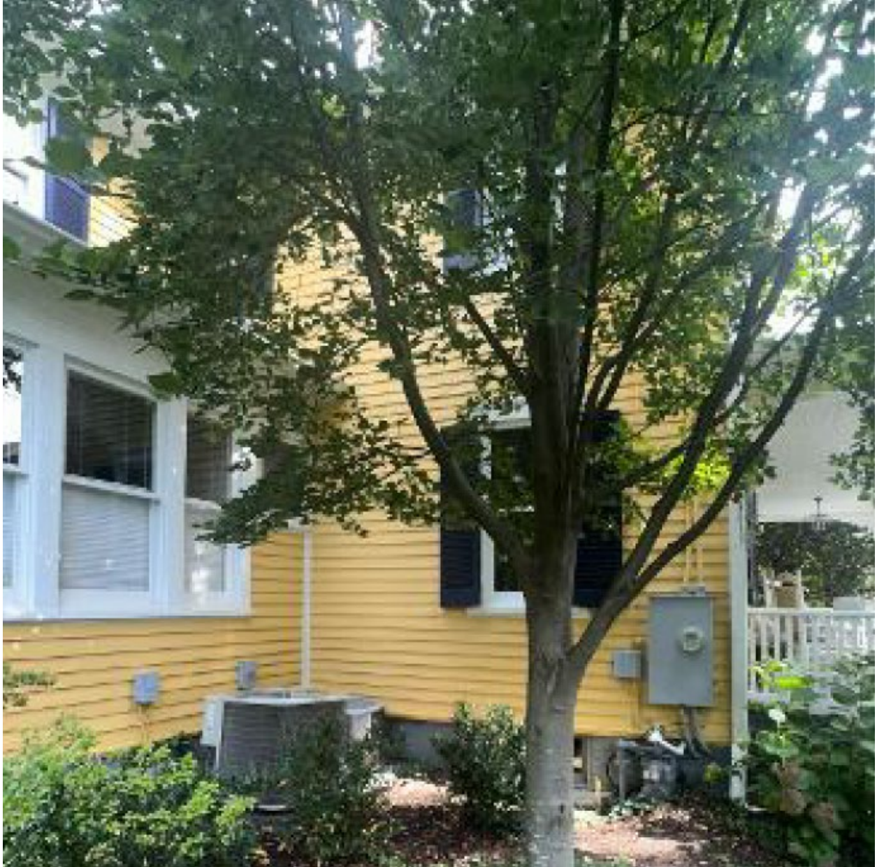
Utility Meter beofre Install
