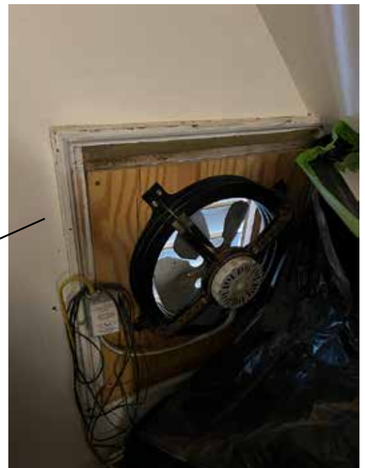
Right window frame (siding on outside of house has been peeled back for a vent for this fan which has been stuck in the window frame)
