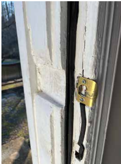
Frame appears to have been altered in multiple ways in unsuccessful attempt to fit door in. Locking area tenuously installed in a crack. Cutout has been made to try to make enough room next to the knob to use it from the outdoors (it is still so close to the frame that it is difficult)
