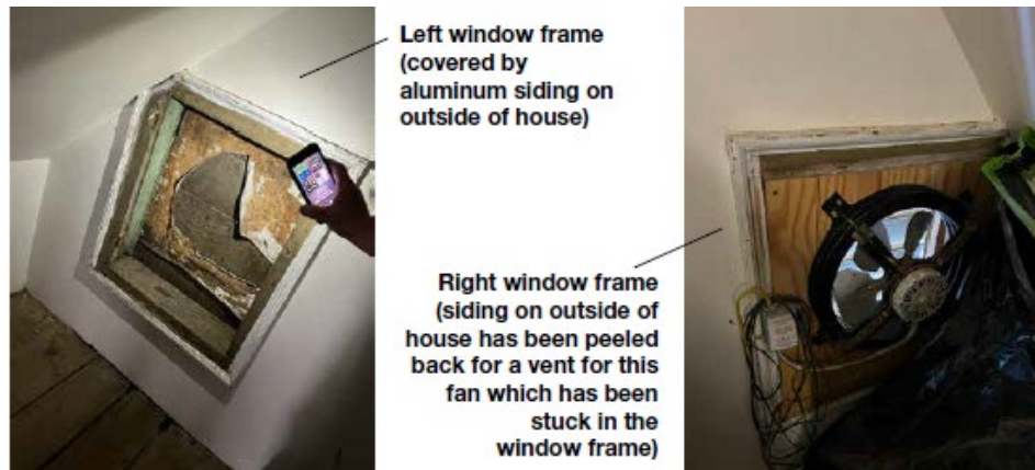
Figure 9: Interior views of the attic windows to be reinstated on the east elevation.
