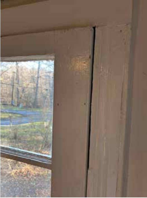
Door sticks out from frame, remaining partially open at the top
