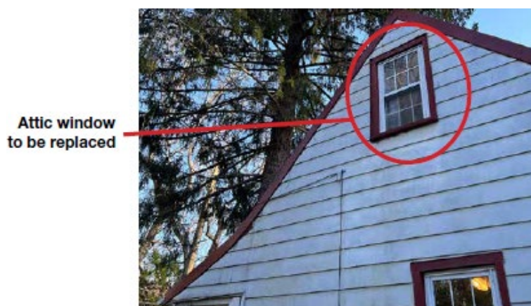
Figure 7: The window to be replaced at the attic level on the west elevation.
