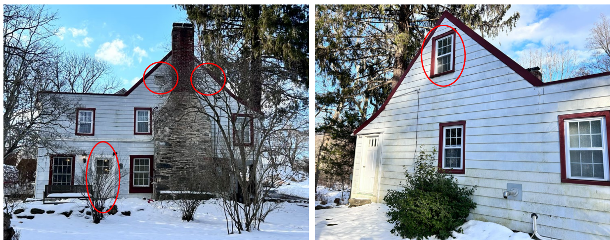
Figure 3: East elevation (left) with locations of door and two windows to be reinstated; west elevation (right) with location of window to be replaced.
