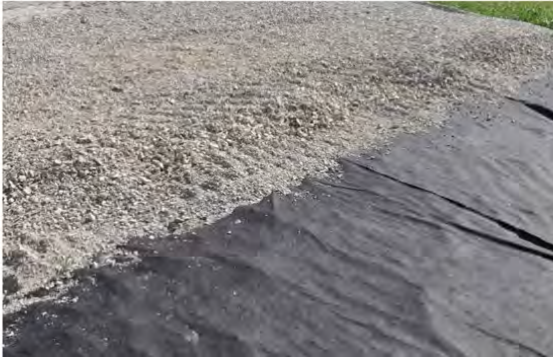
Figure 4: Example image of typical heavy area use pad for cattle. The gravel types of the proposed vehicular use may differ. Source: Perdue Extension, via Penn State Extension.
