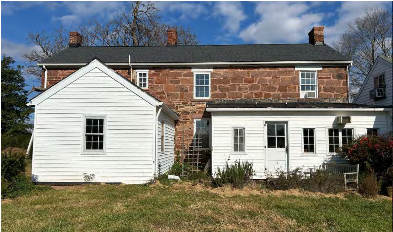
Figure 5: View of the south elevation, including the existing non-historic additions dating to 1954 (left) and 1938 (right). A portion of the gable roof of the historic log kitchen is visible on the right.
