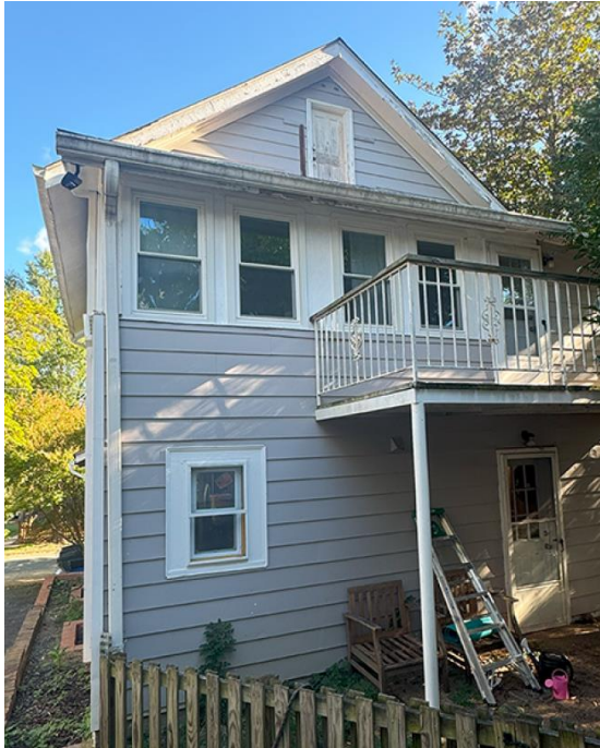
Figure 2: Photo of the rear elevation with the window to be altered circled in yellow.
