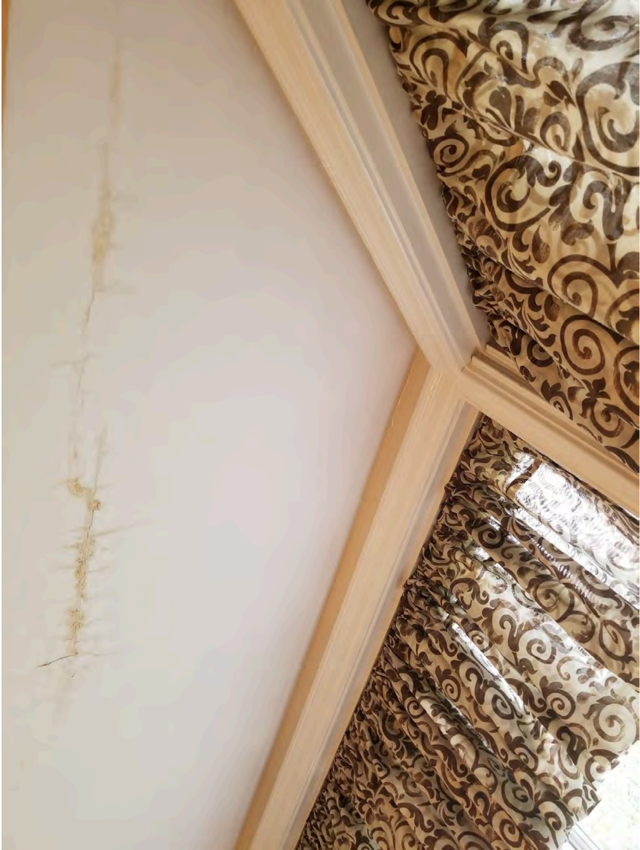
Interior water intrusion from leaky roof over rear bay window
