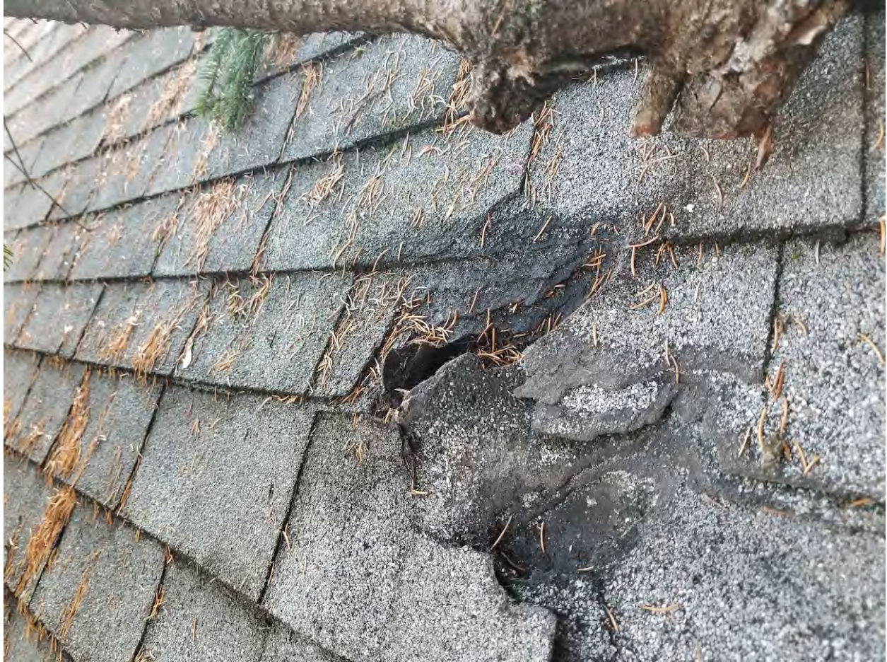
Shingle damage near the northeast corner of the roof caused by a spruce tree branch
