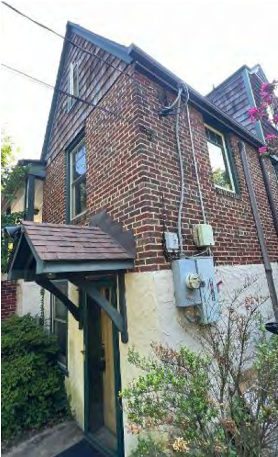
Utility Meter Before Install
