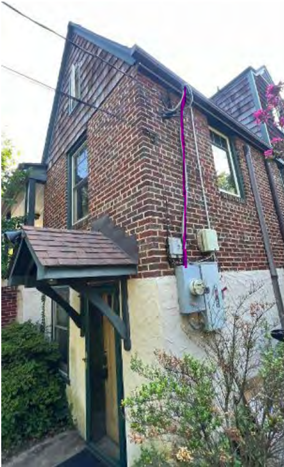
Utility Meter After Install
