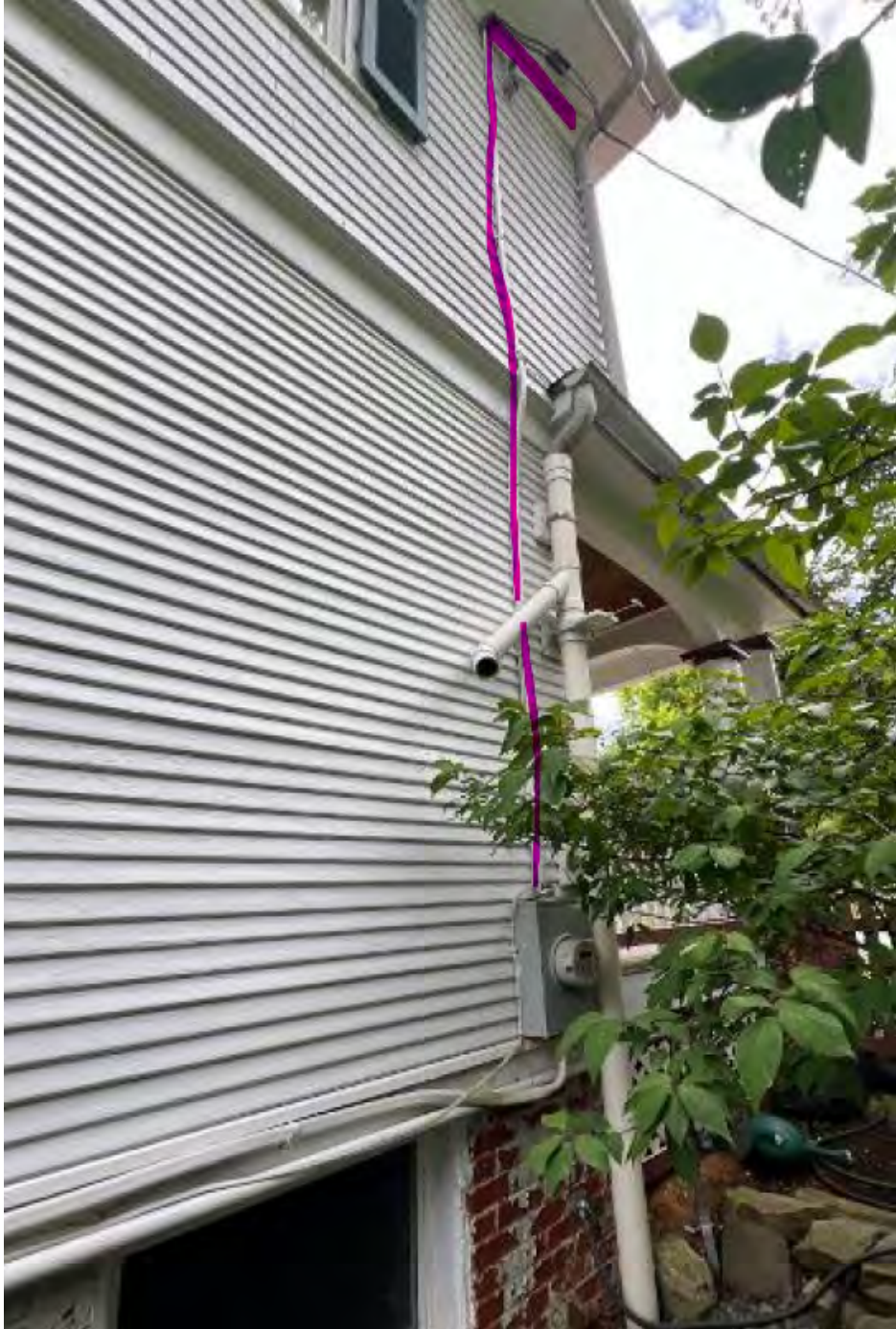
Utility Meter after Install
