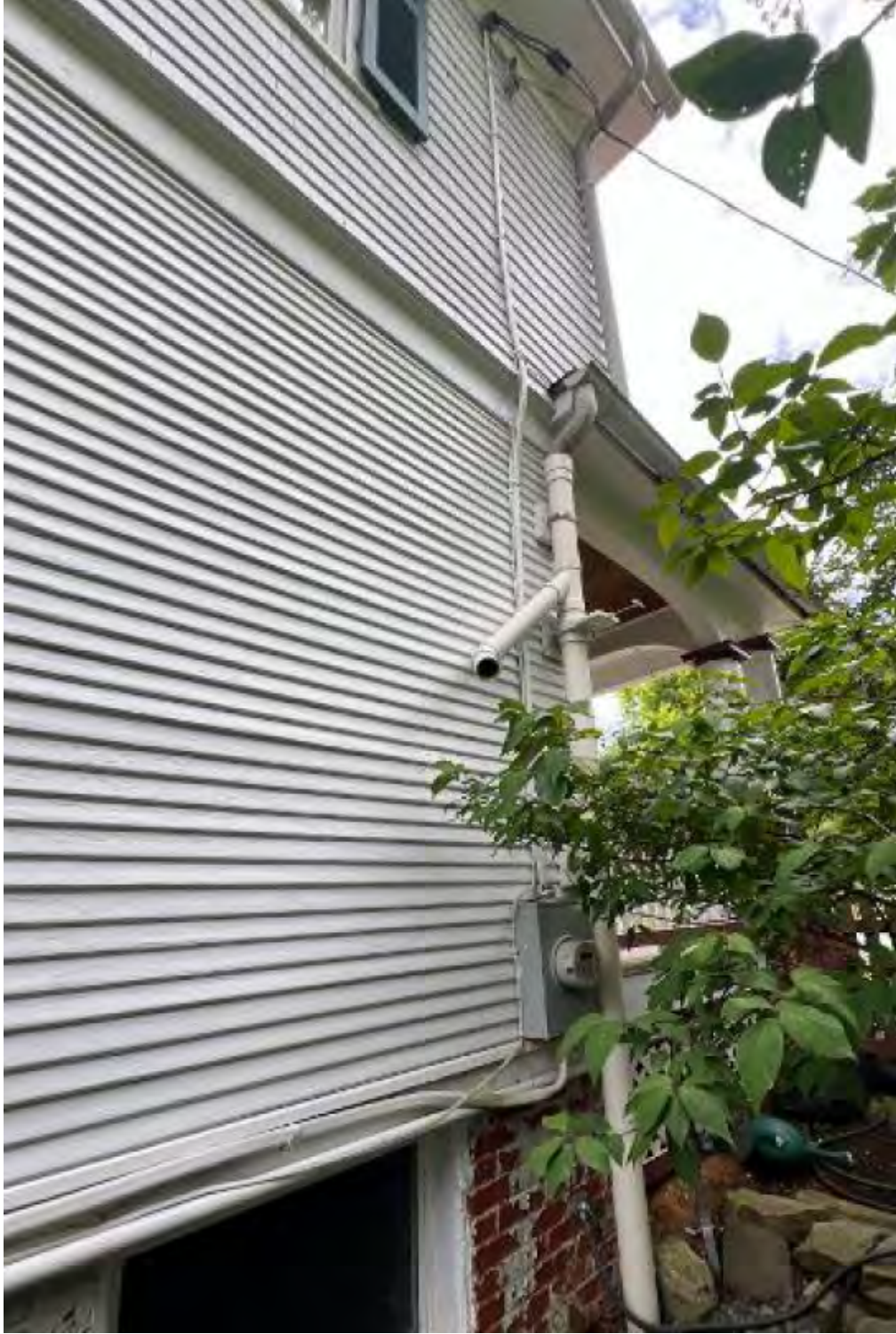
Utility Meter before Install
